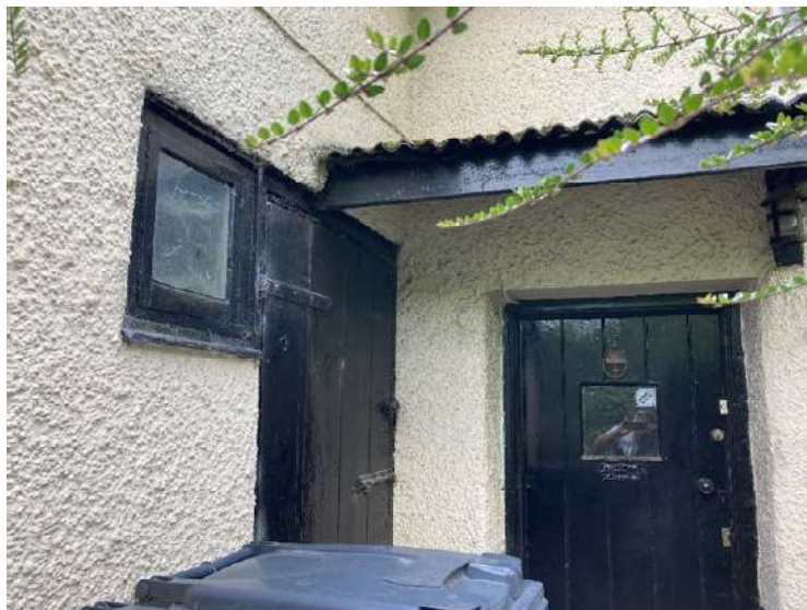
Detail of East facing element of cottage 2 facing the road with entrance door porch and later outside store on the left of the image.
