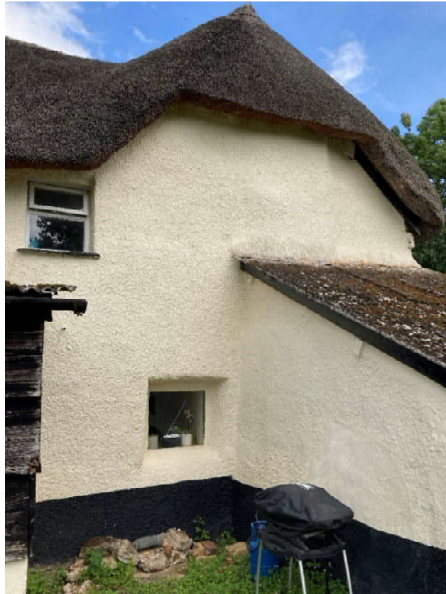
Detail of West facing element of cottage 1 showing end half gable and lean to.
