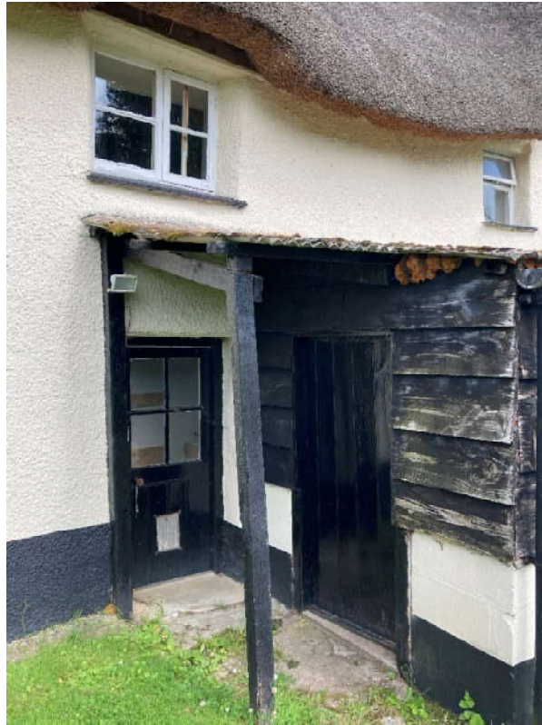
Detail view of cottage 1s West facing rear door and outside porch and store (later addition)
