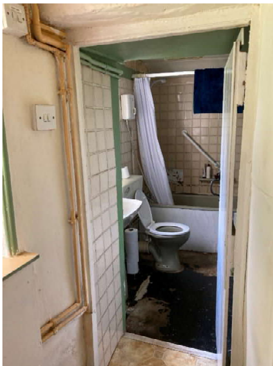
Cottage 1 – Ground floor bathroom in West facing lean to. Viewed from kitchen located in original hallway.
