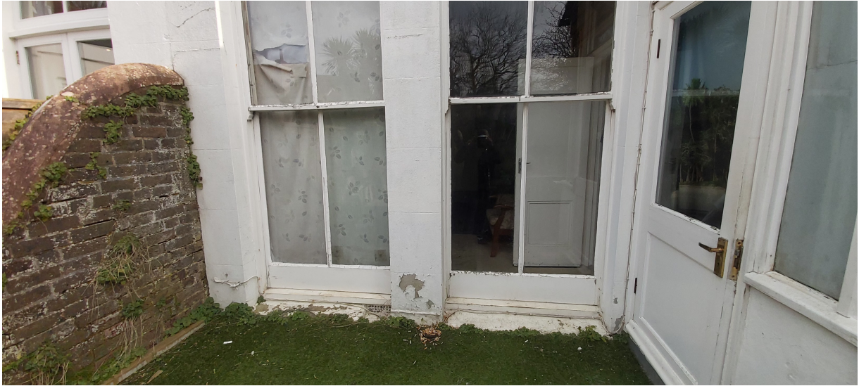
Figure 4 - Existing Rear boundary wall in the vicinity of the proposed conservatory. This will not impact on the neighbouring dwelling.
