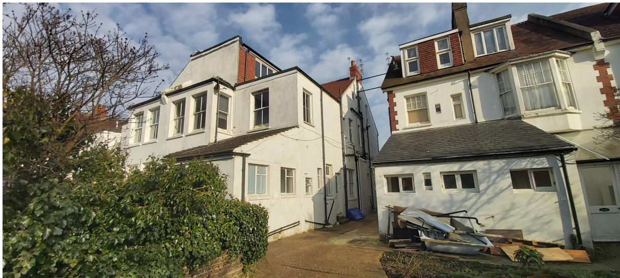
Figure 3 - Existing Rear Elevation showing rendered walls and existing rear dormer set back from the boundaries. The proposed roof balcony, which is set back, will therefore not impact the neighbouring dwellings in terms of privacy and overlooking.
