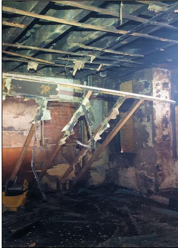
Plate 11: Fire and water damage throughout much of the first and second floors was apparent – here missing a window allowed further access to the internal spaces but there was no evidence of bat activity.
