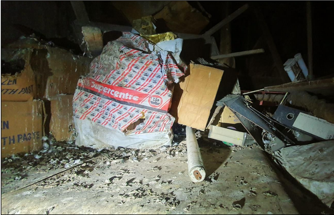
Plate 9: The flat surfaces within the loft void had no evidence of bats. There was considerable evidence of pigeon roosting.
