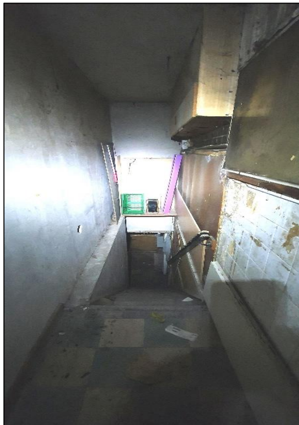
Plate 12: Open doors throughout the building allowed unrestricted access from the second floor to the ground floor; however, there was no roosting potential or evidence of bat activity.
