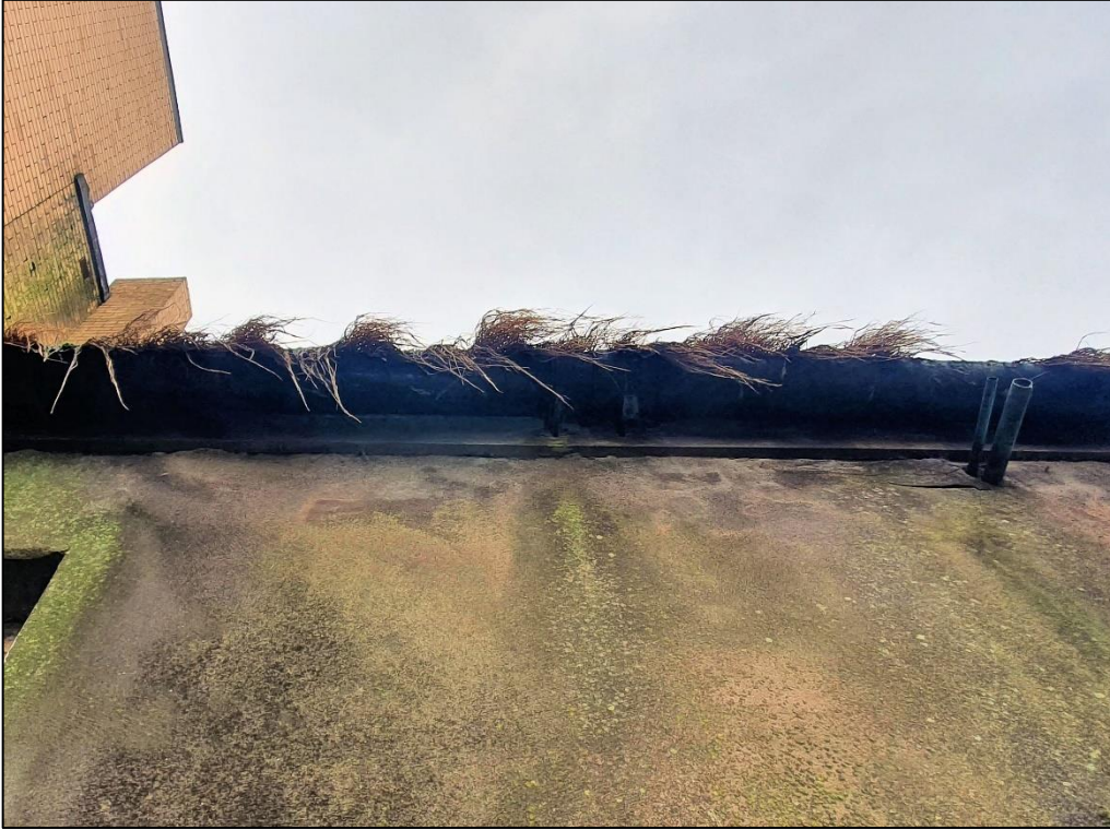
Plate 4: The fascia at the rear of the property was found to be generally intact with no roosting potential.
