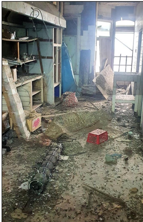
Plate 10: Missing windows and holes in the ceiling allowed access to the rooms on the first floor but there was no evidence of bat activity.
