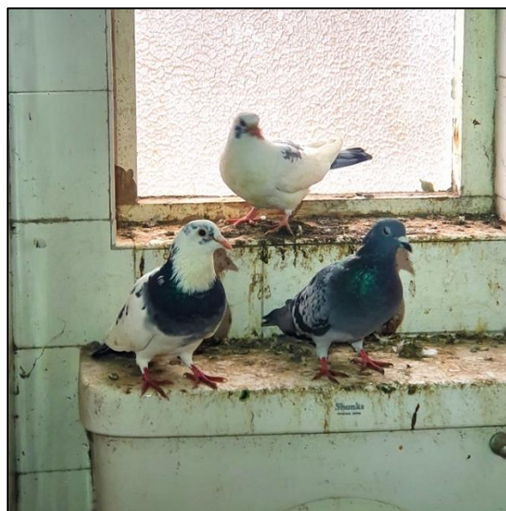
Plate 14: Pigeons were found to be roosting throughout the building.
