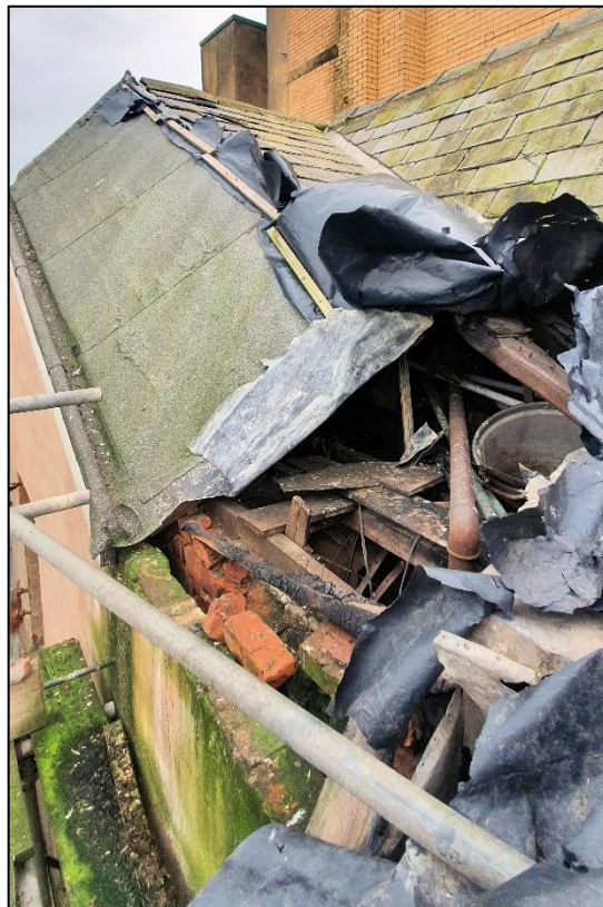
Plate 3: A large hole was apparent on the north west corner of the roof.
