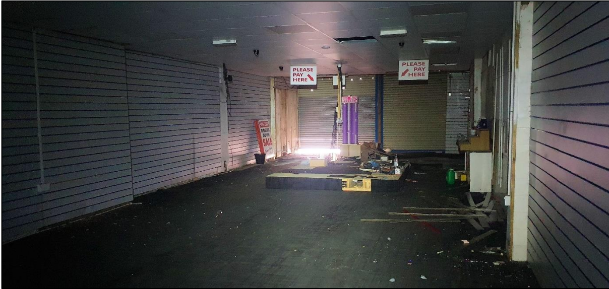
Plate 13: The walls and flat surfaces on the ground floor had no evidence of bat activity.
