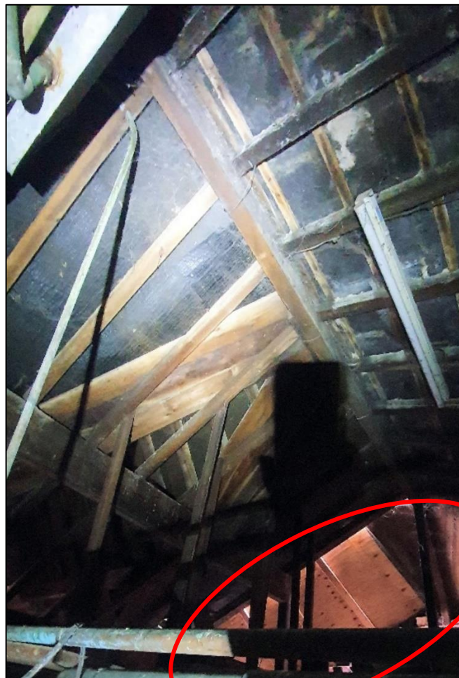
Plate 8: The underside of the tiles or roofing membranes and roof support structures were visible within the roof space; unrestricted access from the outside was possible via the gaps in the roof (red circle).
