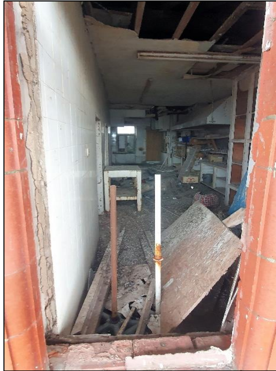
Plate 6: Missing windows and window bards at the front of the building allowed free access to the internal spaces.
