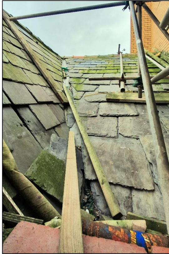
Plate 2: The roof was in poor condition with gaps under and between tiles.
