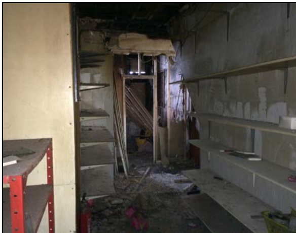
7. Internal view of the front portion of the first floor of No. 86 Promenade confirming no features of historic interest remain.
