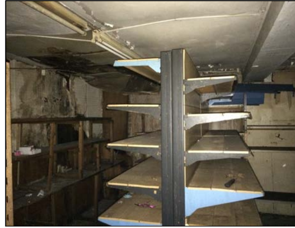
6. Internal view of the rear portion of the first floor of No. 86 Promenade confirming no features of historic interest remain.
