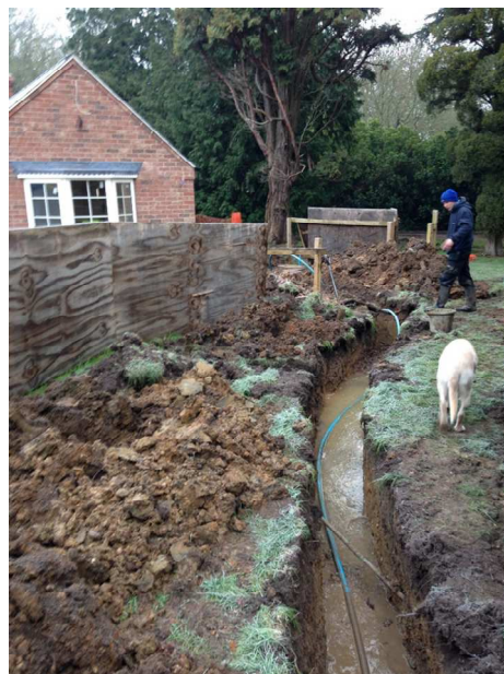
Photo 2 (provided by client): Historic ground works undertaken to the south east of the bungalow
