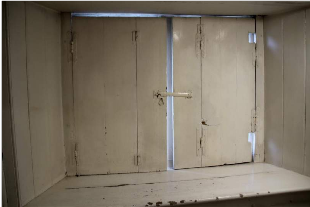
Photo 32. Plank shutters to the small window to the basement stairs, with original ironmongery
