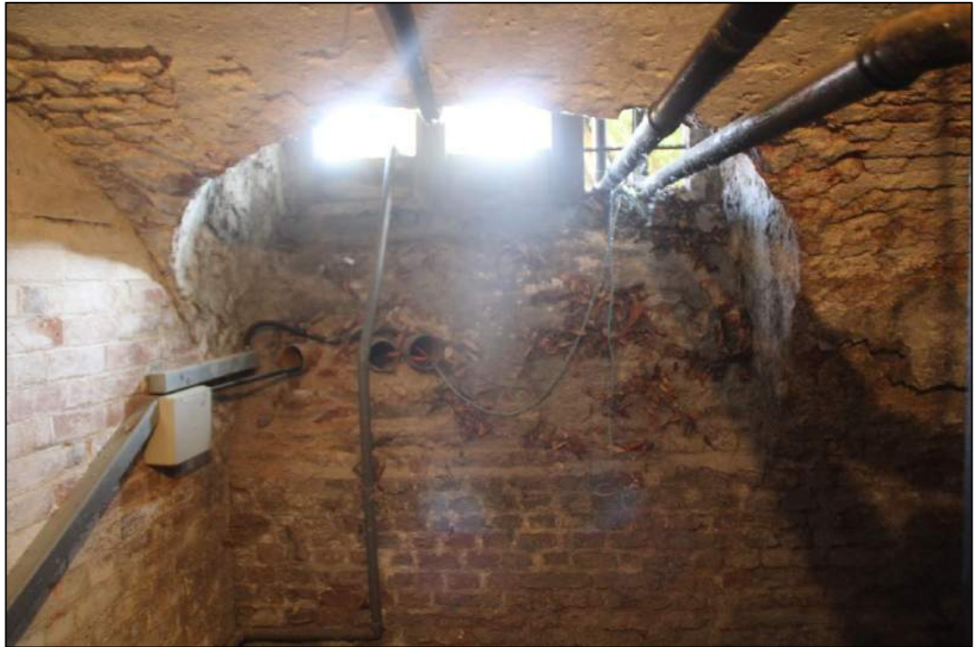
Photo 42 Interior view of the mullioned ground level window seen in the stable courtyard, in Room B4
