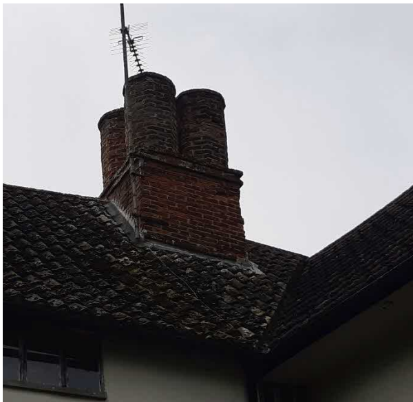
Photograph 2: Back of house, lifted lead flashing at base of chimney
