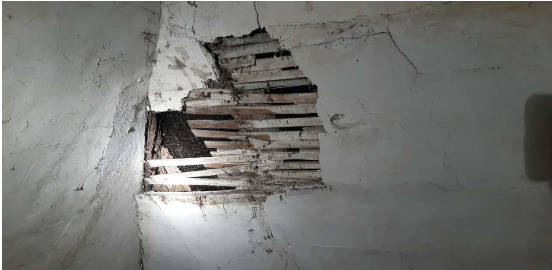
Photograph 4: Room at the eastern part of the loft, broken plaster
