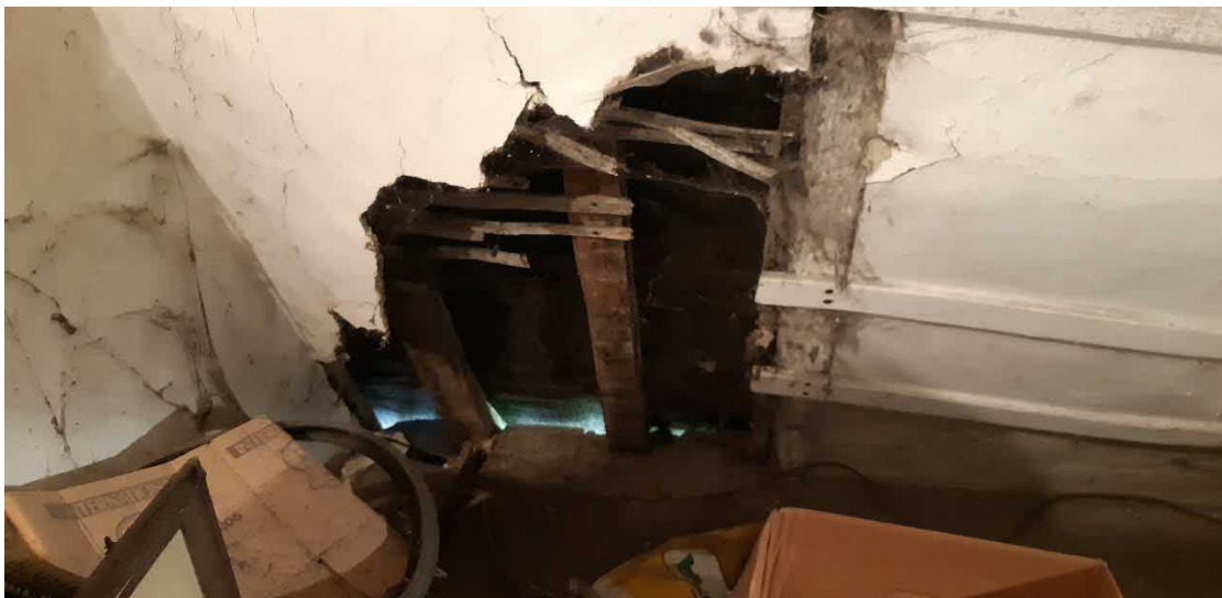
Photograph 5: Gap in the eaves in the eastern room
