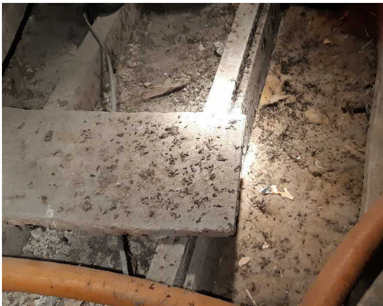
Photograph 7: A cluster of bat droppings, western loft space
