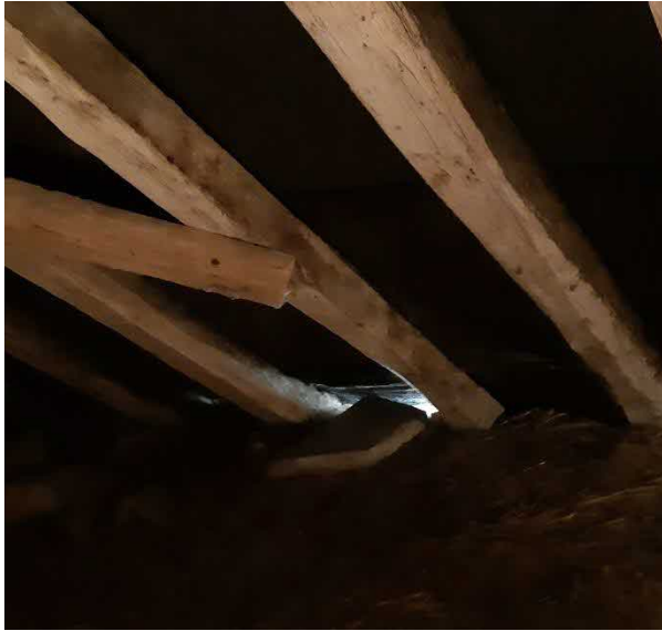
Photograph 3: Gaps at the eaves, western loft space, providing easy access
