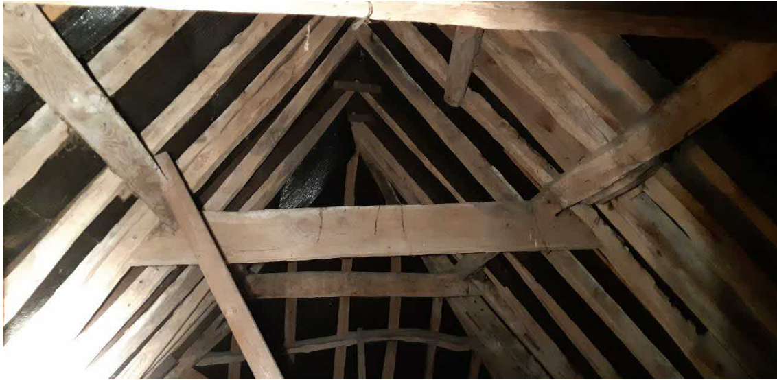
Photograph 6: The void in the western loft space
