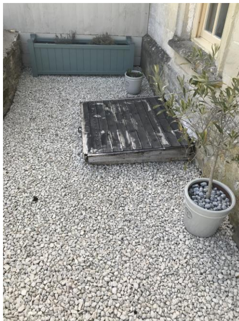
Figure 1: Decayed external cellar hatch to be replaced with glazed side hung hatch.
