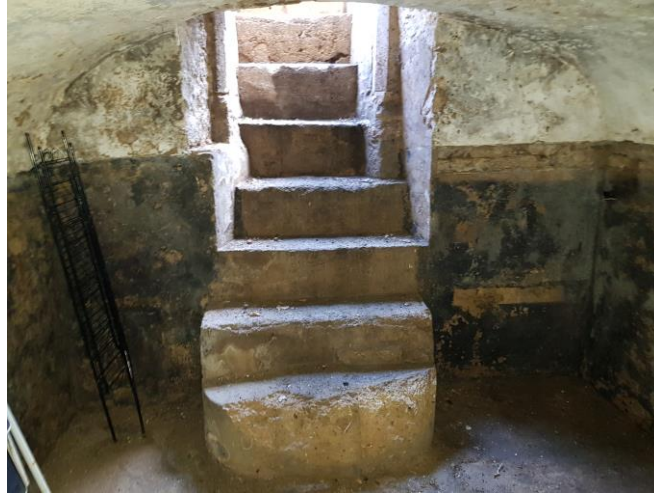
Figure 2: Steps down to the cellar. Proposals seek to remove the bottom two steps to provide additional storage space.
