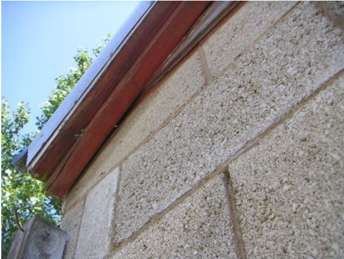
Photo 12 – Example gaps where the wooden boxed soffit meets the wall on Building 9.
