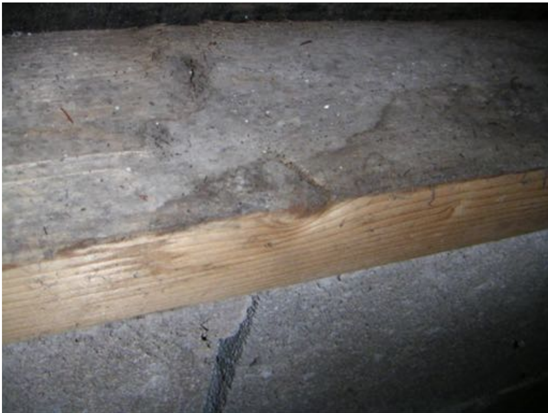
Photo 30 – View of gap where mortar is missing between breeze blocks on wall within the northern section of Building 10.
