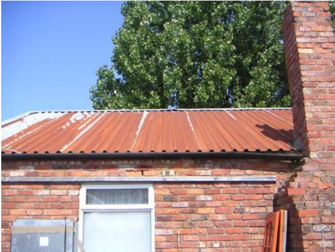
Photo 13 – Southern aspect of Building 9, gaps in brickwork which were fully inspected and found to be superficial.
