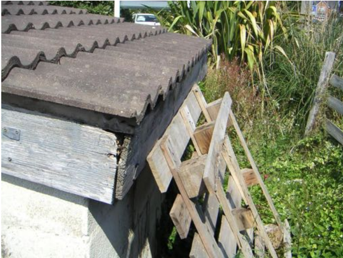
Photo 3 – View of gaps in the wooden barge boards on the southern and eastern aspects of Building 2.
