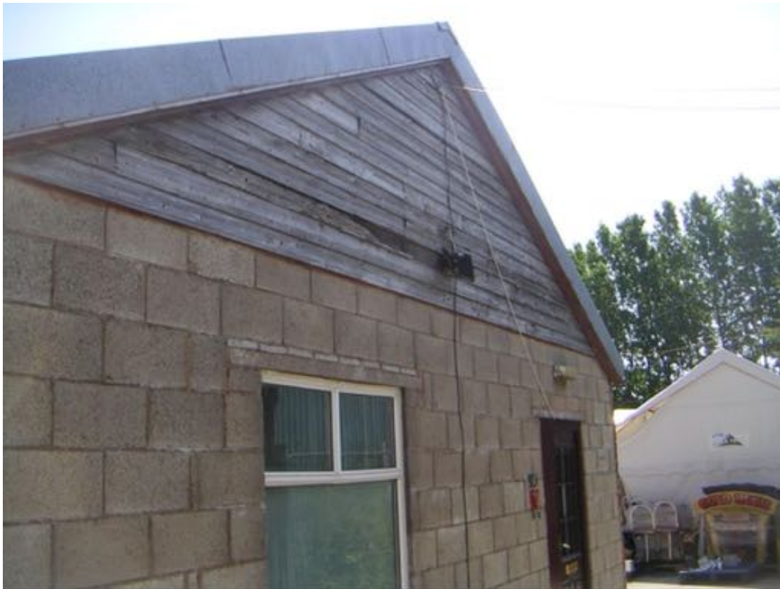
Photo 11 – Western aspect of Building 9, view of wooden boxed soffit and wooden cladding.
