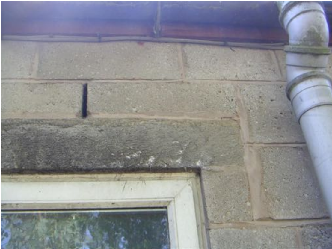
Photo 14 – Northern aspect of Building 9, with one gap recorded in where mortar is missing.
