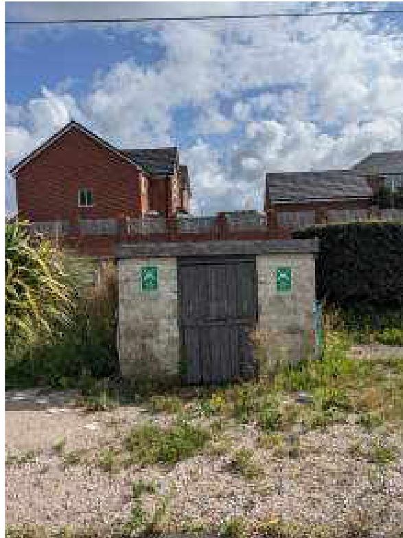
Photo 16: View north east showing meter gas and electricity meter units in the north eastern corner.
