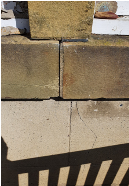
stone mullions moving and unaligned as a result of damage to principle masonry wall
