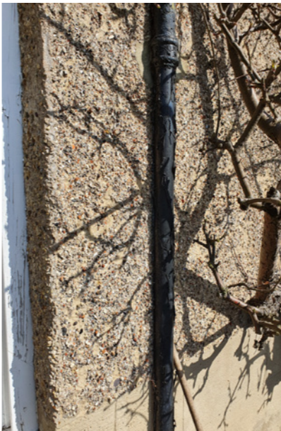
existing downpipes buried within render, pipes rotting and failing causing damp internally
