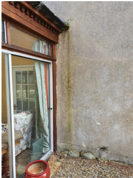
dated conservatory at end of life, leaking at abutment causing further damage to render
