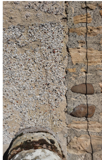
existing stonework splitting, poor quality pebble dashed render
