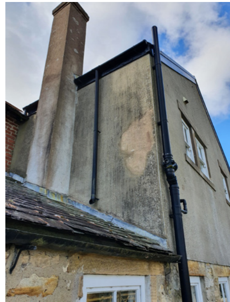
failing concrete render causing damp problems internally
