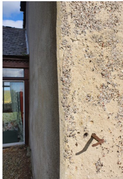
Poor quality render, pebble dash failing and cracking
