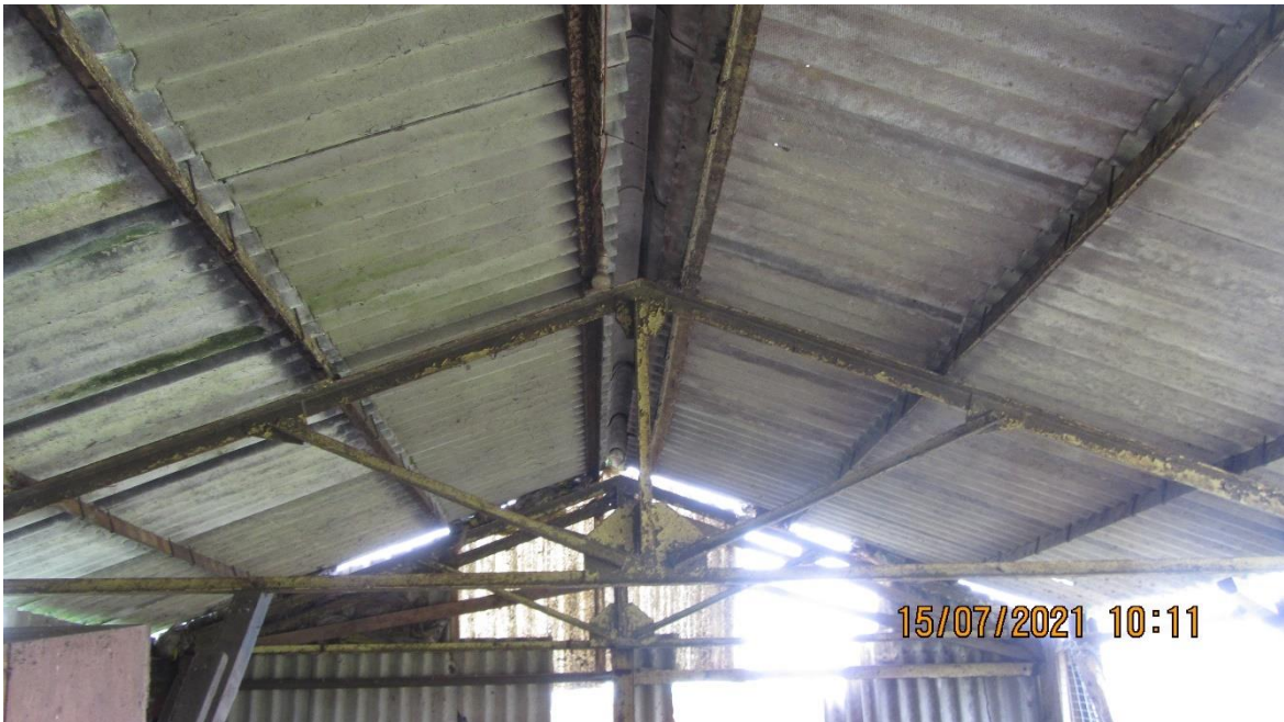
Photo 10. View of the interior of the barn with no enclosed roof space
