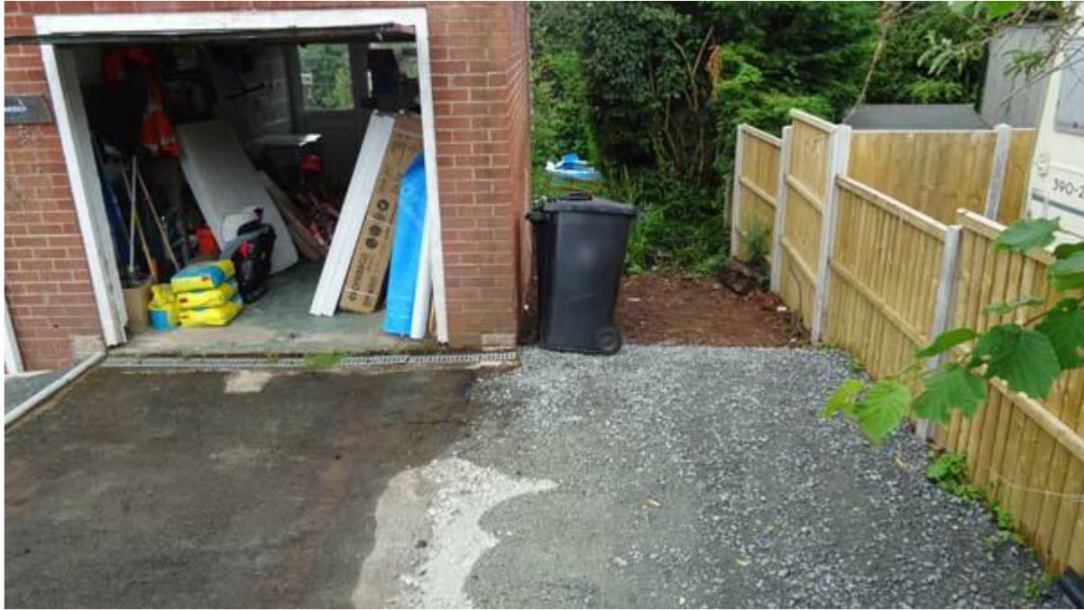
DETAIL OF THE SIDE SPACE TO THE WEST BOUNDARY – New garage increase in width to the refuse bin leaving 1300mm gap for a side gate between the new masonry and the fence panelling. The adjacent property is set away from the boundary with existing side driveway and parking area.
