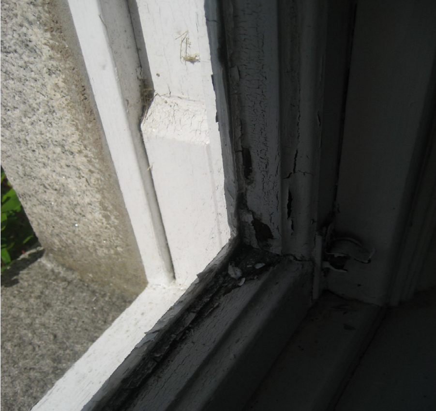
The existing frames are rotten through and are beyond repair.
