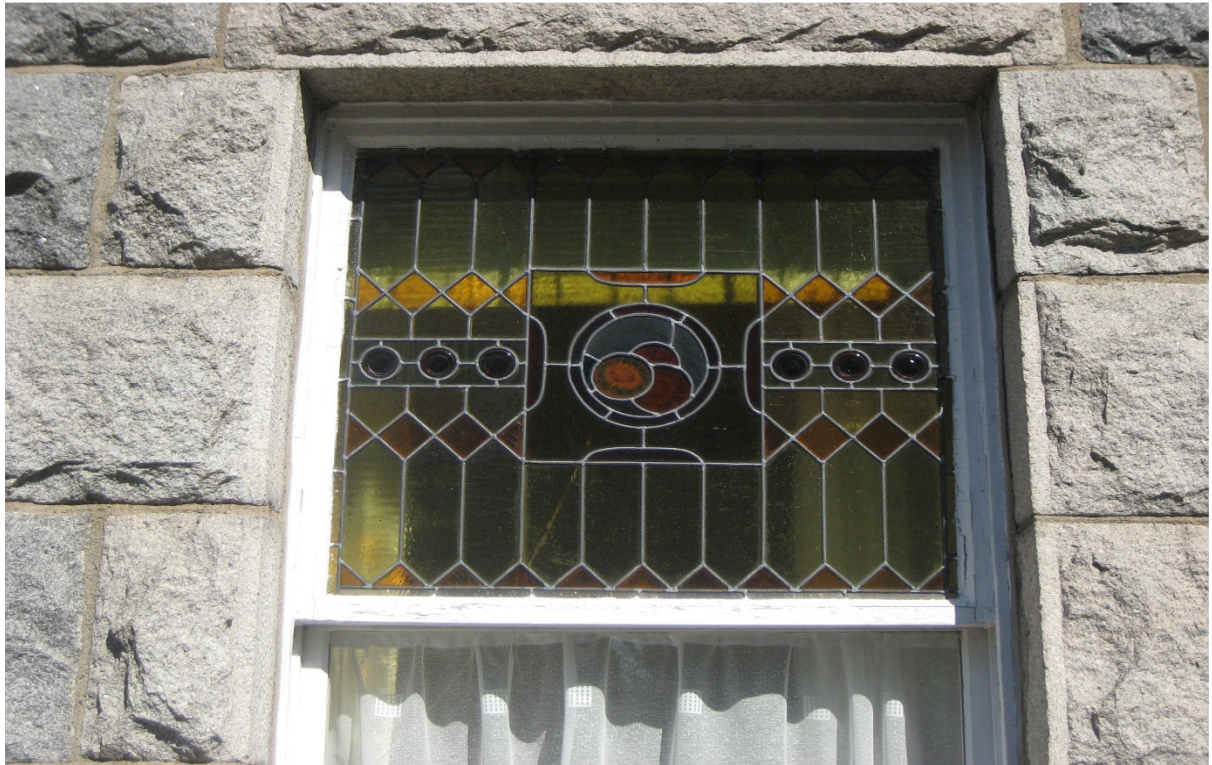
Existing Bedroom (W4) Window showing the existing Lead detailing. The lead detailing is going to be carefully removed from the existing sash and placed within additional new frame (not within the new sash) that will sit inside the new windows
