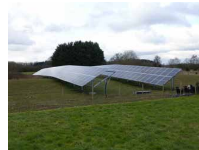
Shropshire Council are now committed to zero carbon and will utilise solar energy wherever possible.
