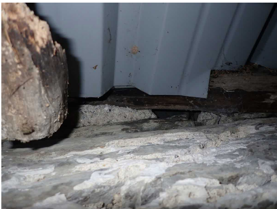
Photo 9. Example of a crevice suitable as a roost access point where the roof of the lean-to shed met the house gable wall.
