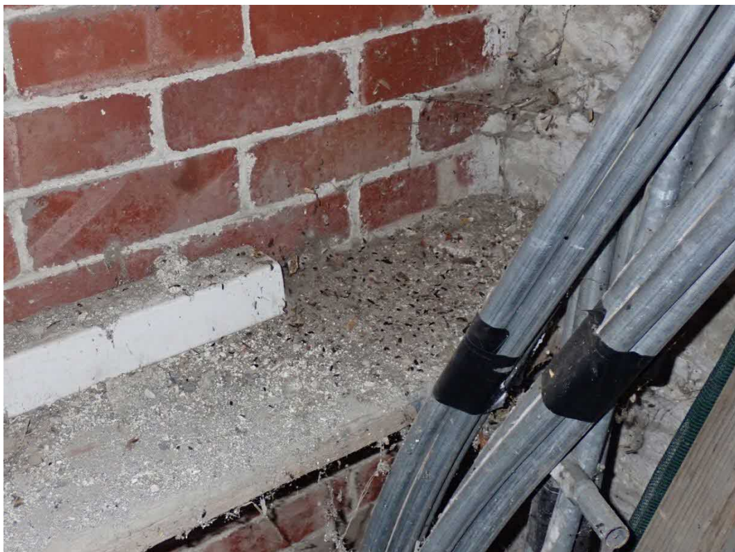
Photo 8. Group of droppings on a shelf in the lean-to shed next to the SW gable wall of the house, probably indicating a day roost above.
