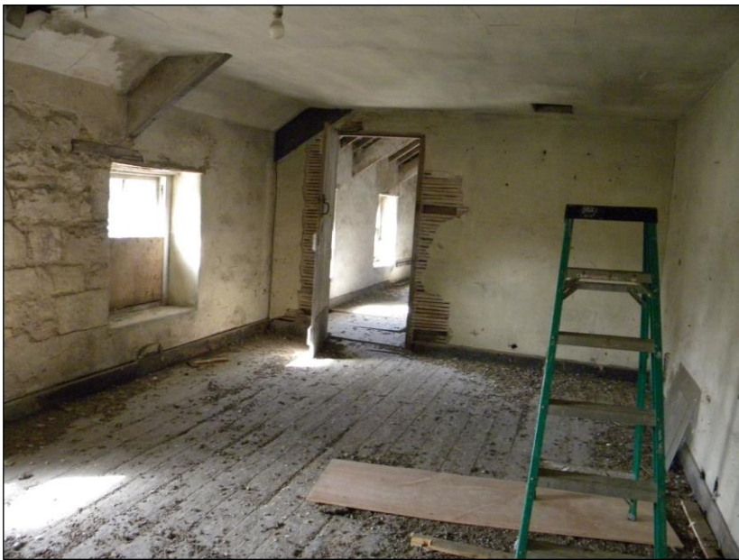
Figure 23. Large room to middle section upper floor with pigeon evidence above stables.
