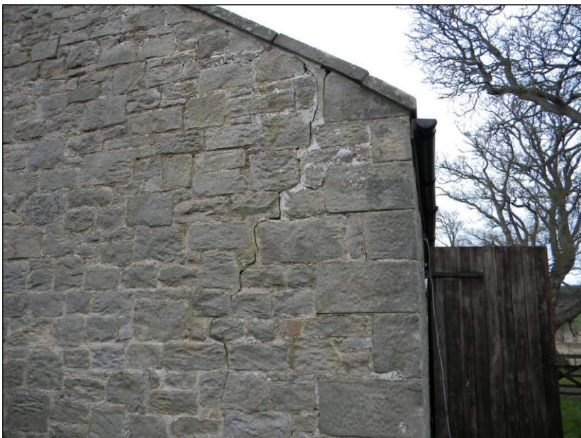
Figure 33. Gaps in stonework/pointing to the cartshed and underneath water table.
