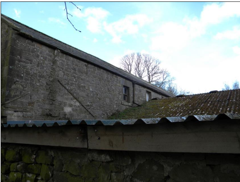
Figure 14. Rear (north east) elevation of stables adjoining land not in the ownership of the client.
