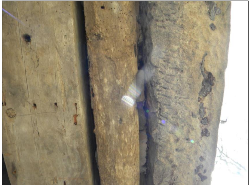
Figure 16. Stables - gap above door lintel lower floor stables.
