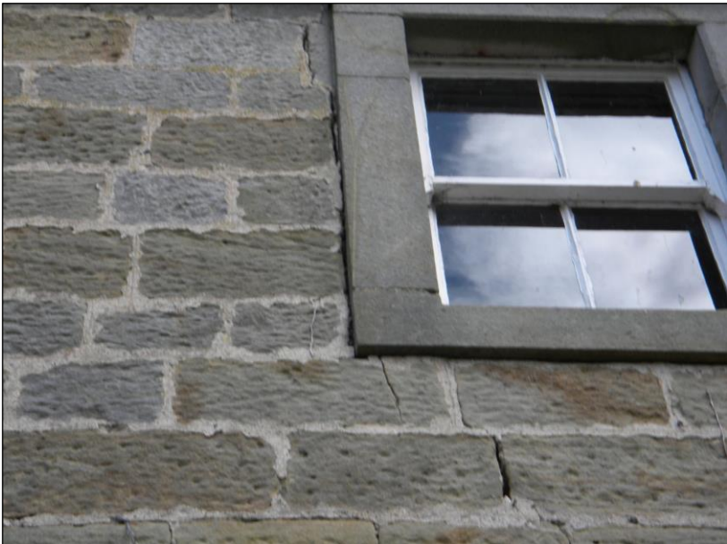
Figure 12. Gaps around stone window surround of the upper floor of the stables.
