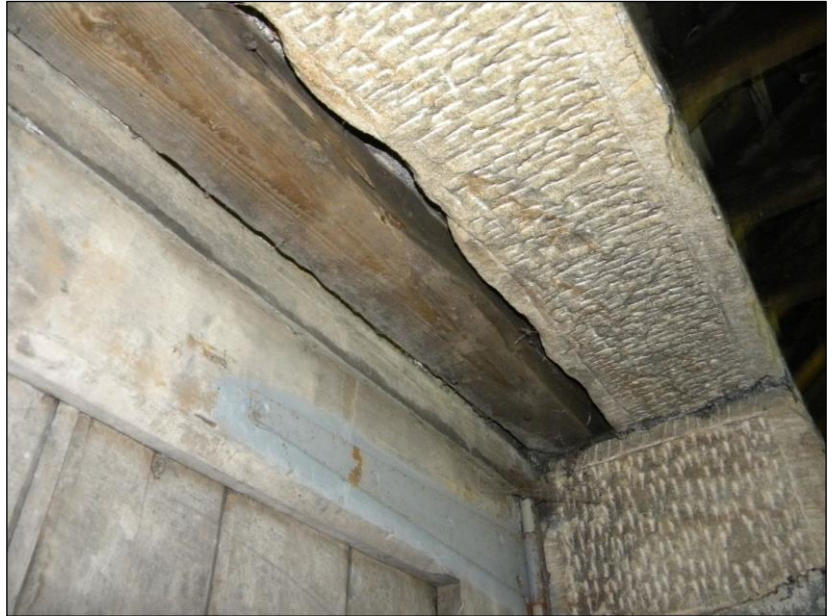
Figure 34. Internal cartshed – gaps around stone lintels.
