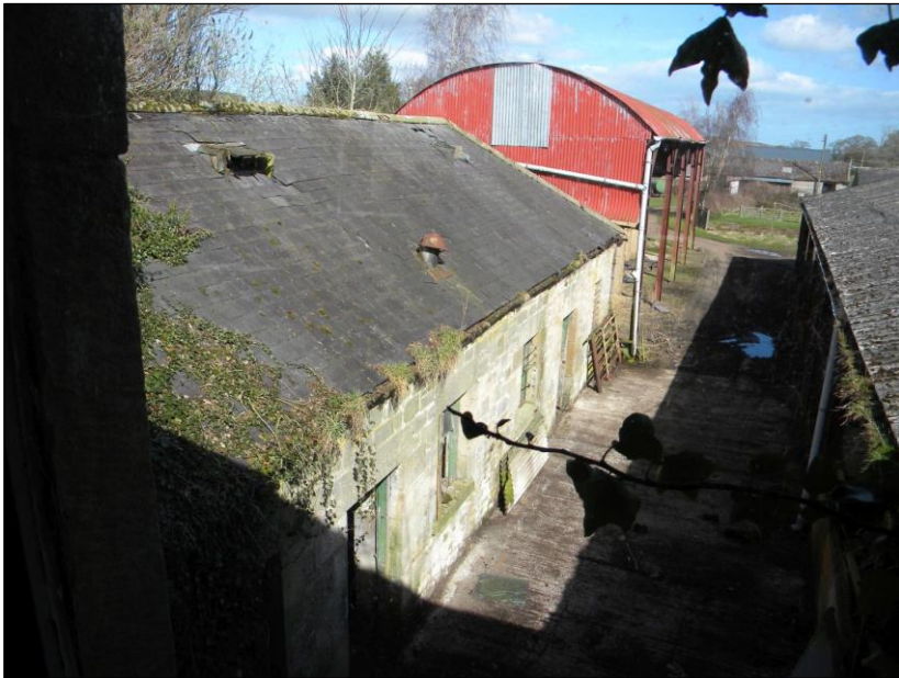
Figure 25. Buildings to rear not in ownership of client but may be looking to buy/survey. Stone building not inspected internally risk assumed moderate.
