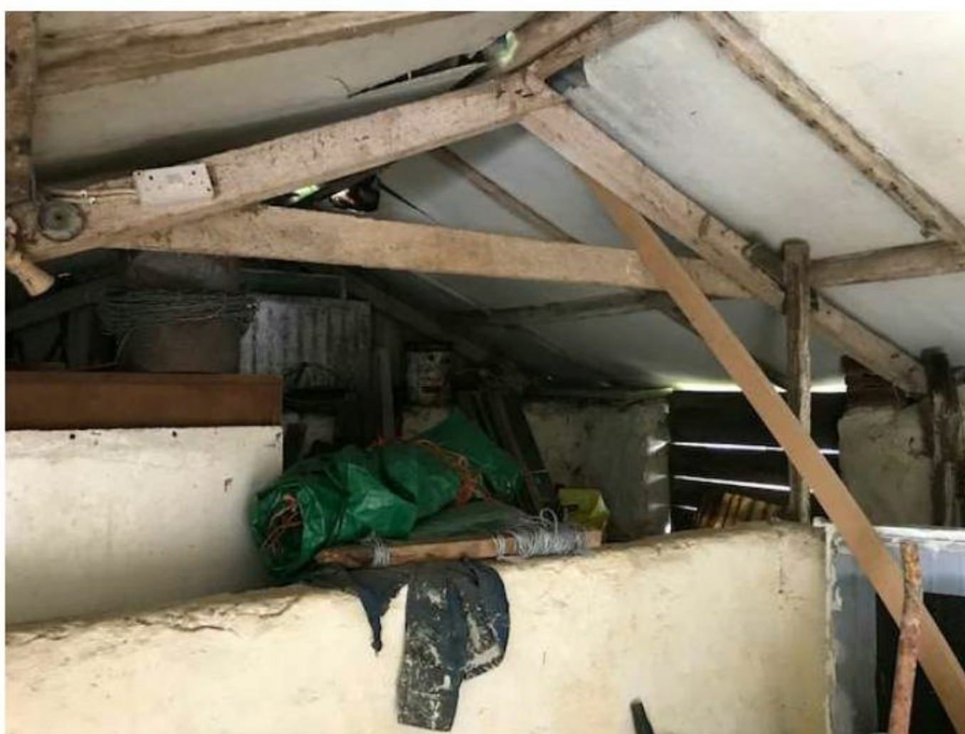
Figure 4: View of interior of the old piggery, showing dividing half block walls.
