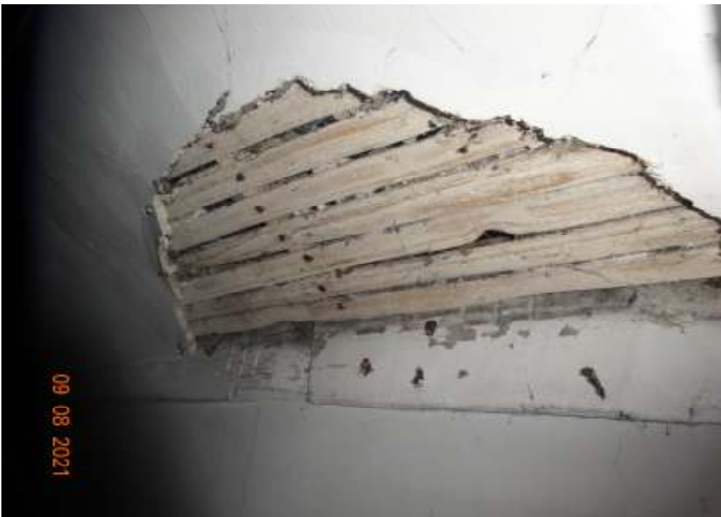
Photographs showing existing damage to Ceiling & Walls to the lathe and lime plaster on the Existing 2 nd Floor.
