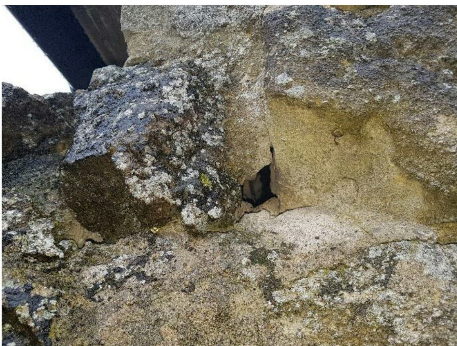
Photograph 5. Gap in the mortar on the eastern face of the dwelling.
