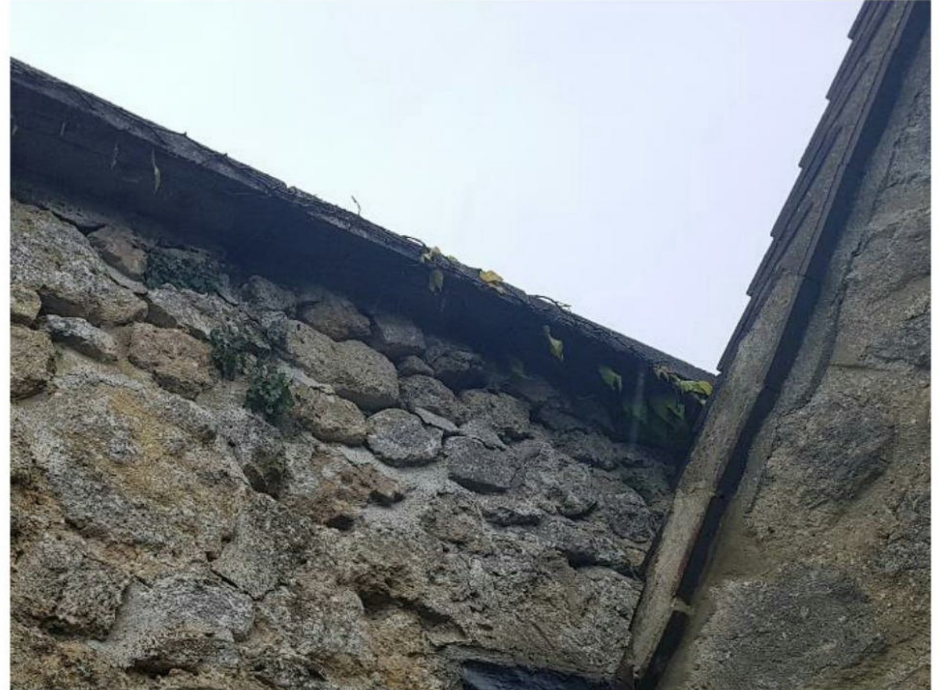
Photograph 8. Gaps between stone blocks on the interior face of the western ruin wall.
