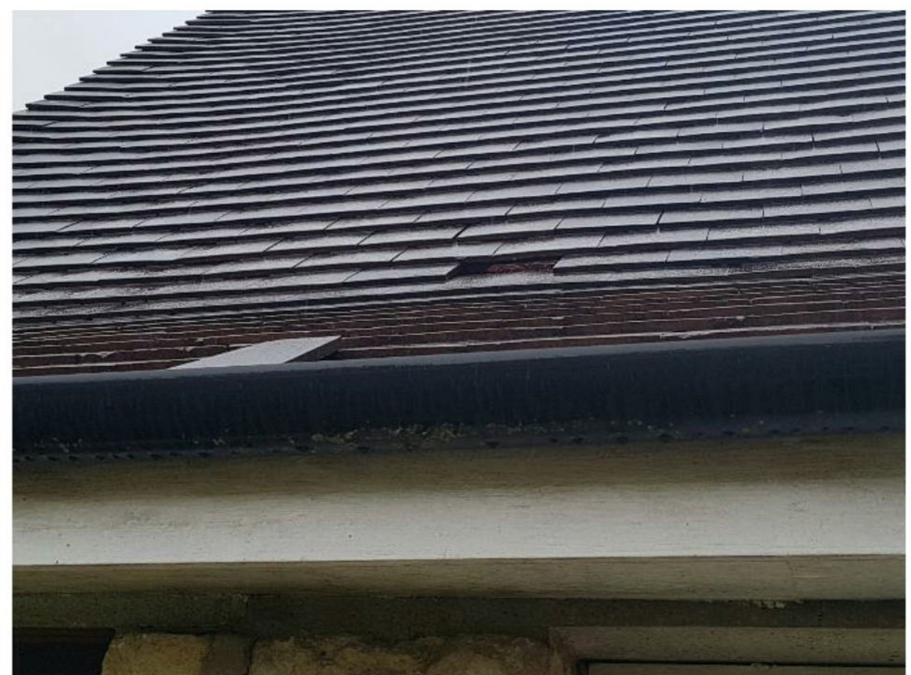
Photograph 4. Slipped tile on the eastern pitch of the dwelling.
