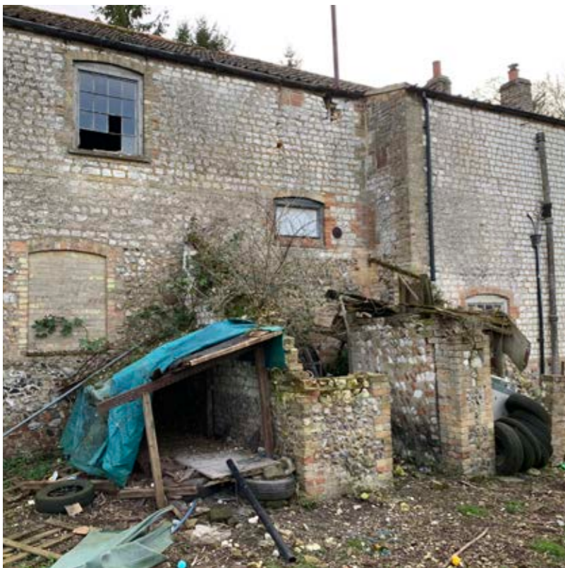
Delapidated lean-to on North Elevation
