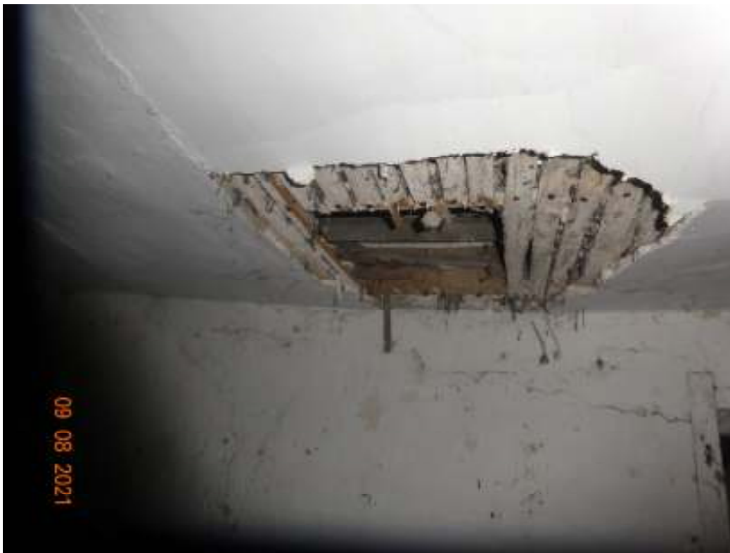
Photographs showing existing damage to Ceiling & Walls to the lathe and lime plaster on the Existing 2 nd Floor.
