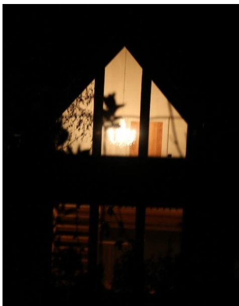
Image 1: The pendant luminaire installed in the staircase of the constructed dwelling. This luminaire is the main source of illumination in this space.
