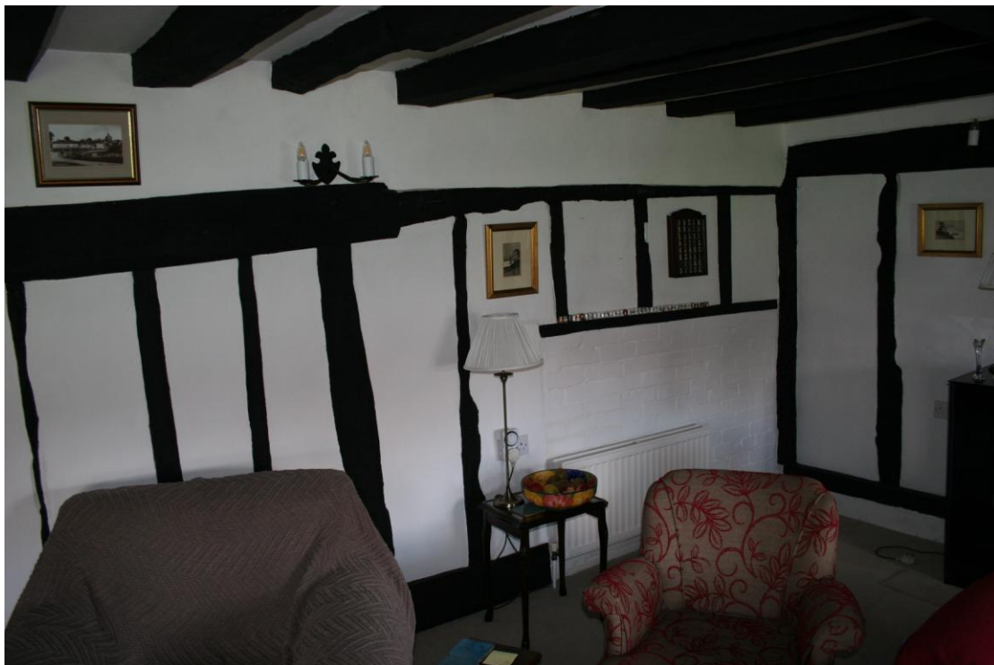
Looking SW in the Sitting Room at the brick wall of a former oven.
