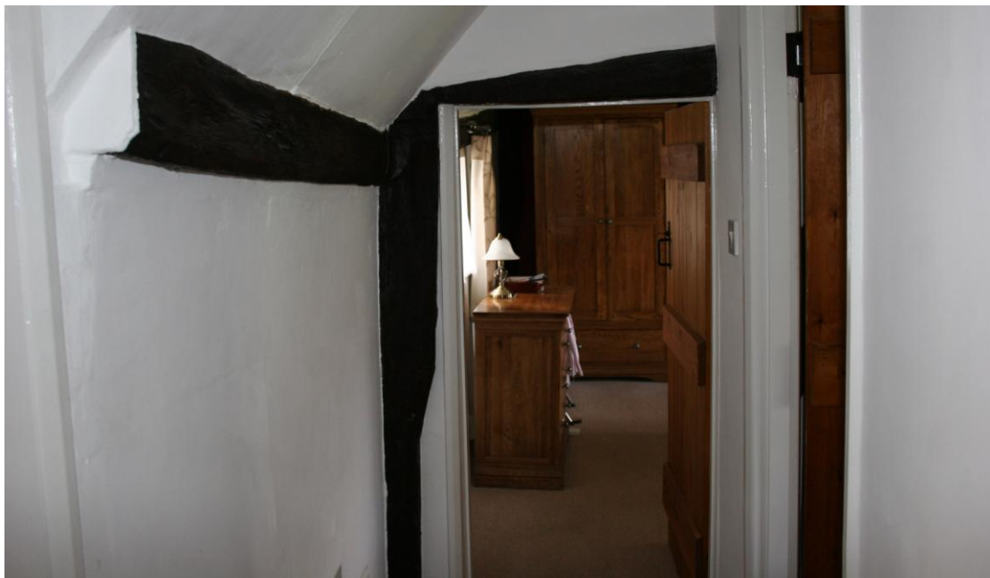
The truss has been cut back to insert the doorway. Looking W.
