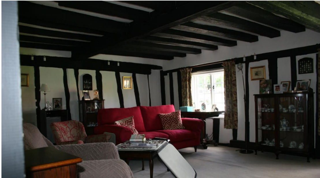
Looking NW in the Sitting Room. Note the cut out for a corner post by the window.
