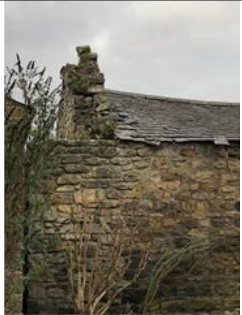
4. Loose stonework to the top section of the gable wall
