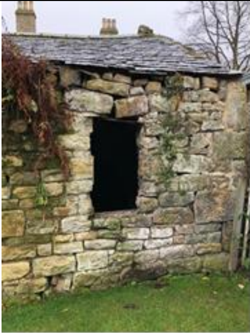
5. Defective stone lintel above the window opening on the rear elevation
