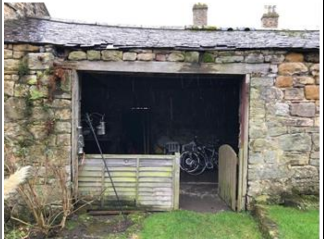
8. Defective timber beam above the large opening on the rear elevation
