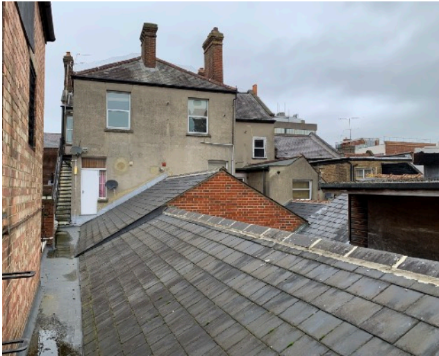
Fig.1 View towards the main building on High Street from the rear. Showing the fire escape from the existing flats to the roof of the rear structure.
