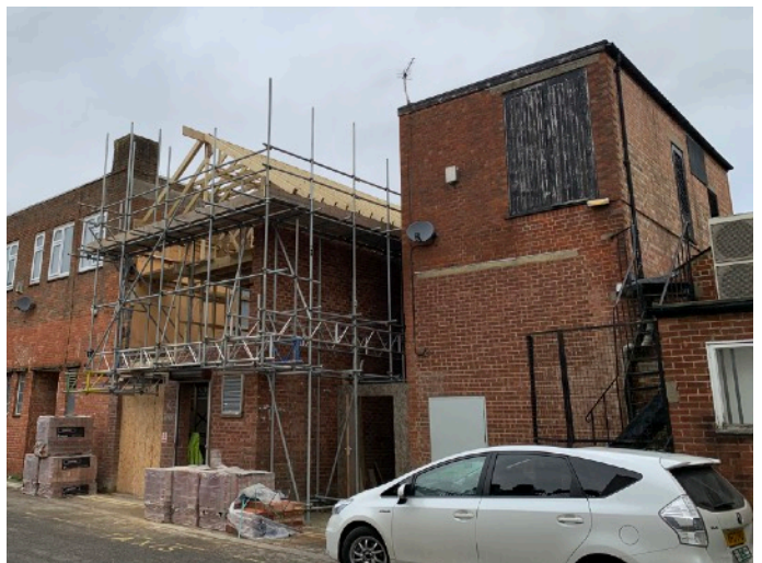
Fig.4 View up Nicholsons Lane, showing the construction of the permitted development 18/03412/FULL and the existing 2 storey portion of 87-89.
