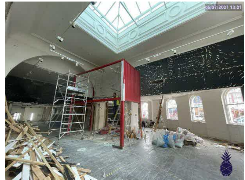
Plate 8: Double-height space looking towards the south and mothballed first floor area beyond the black-painted wall.
