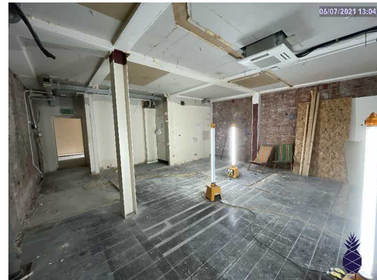
Plate 29: The location of the proposed hoist at ground level with modern structural elements visible.
