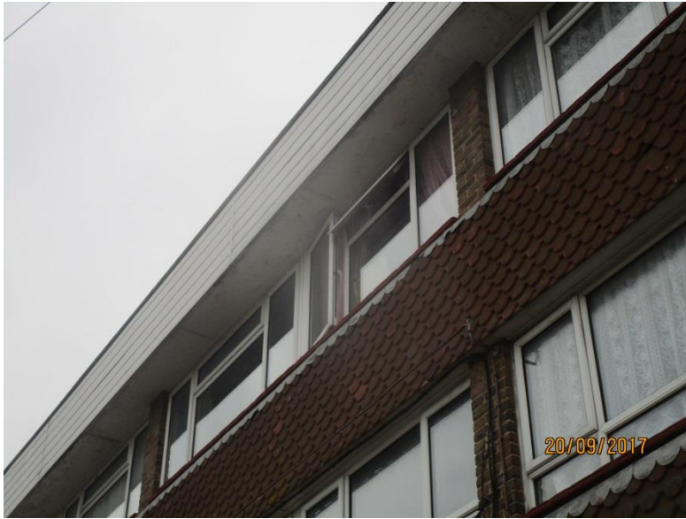
Photo 4 - Existing Facia Board and Soffit
