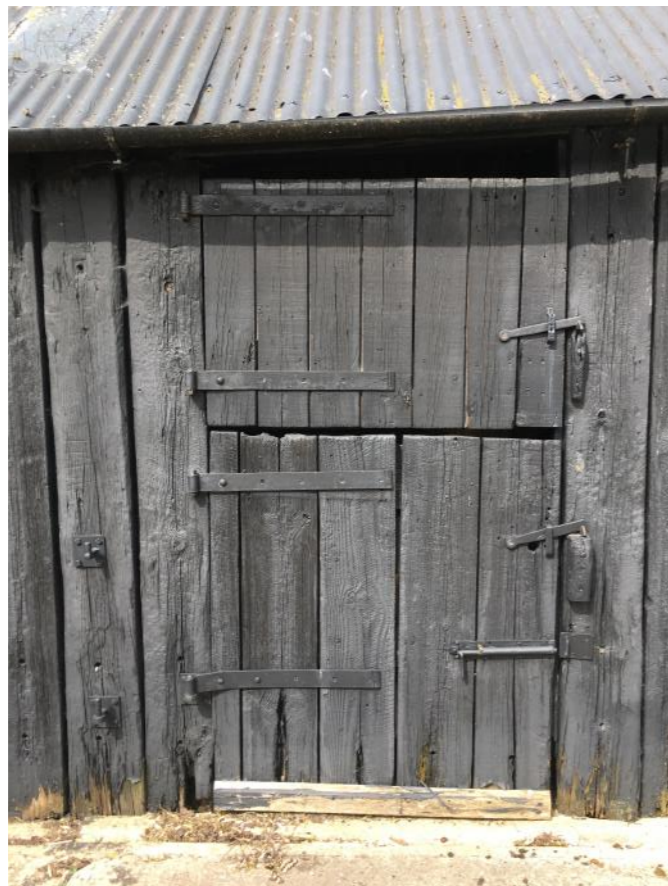
Plate 22: Stables doorway with typical mass produced ironmongery, matched elsewhere on the farm.
