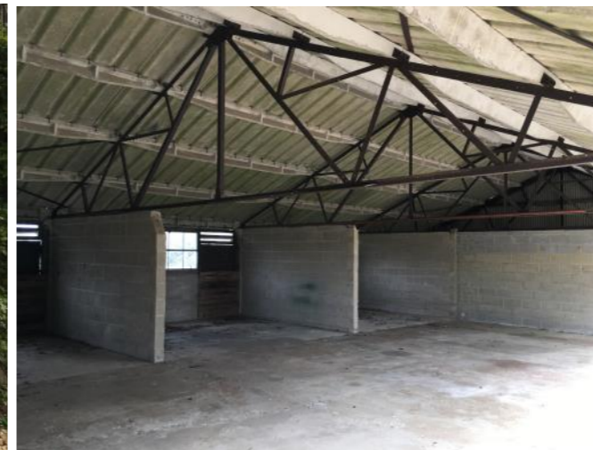
Plate 20: Building 17 interior showing steel truss, modern roof and concrete block walls. Vehicle storage has been most recent use and there remains no evidence or clues to any former animal accommodation function.
