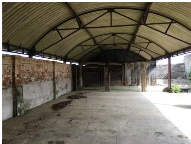
Plate 18: Bow roofed and steel supported storage shed at the rear of the main barn. Formerly location of shelter sheds for animals.
