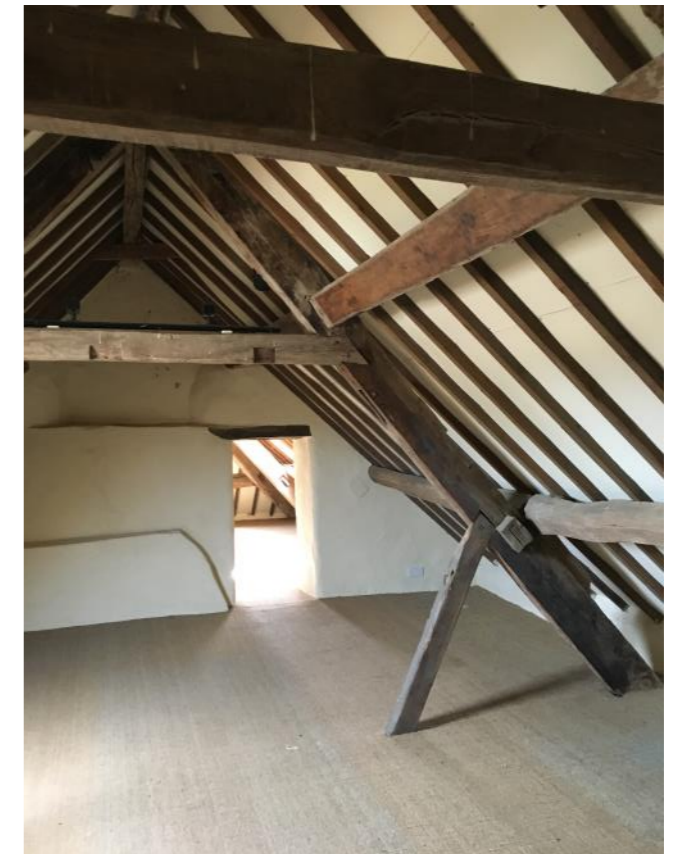
Plate 24: Main roof over the historic core of the farmhouse. Structure shows frequent new rafters associated with the re-roofing, evidence of removed, relocated and raised collars and braces and the re-positioning of the purlins to be lying over instead of butted up to the principal rafters.
