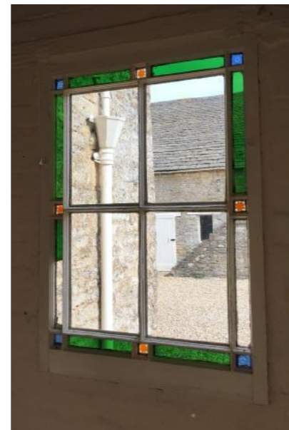
Plate 4-5: (left) early casement set into the stone mullion at first floor, simple turnbuckle catch and loop on the bottom of the casement to take the twisted stay just visible externally. (right) typical mid 19th century window with brightly coloured glass within margin lights; rear porch.
