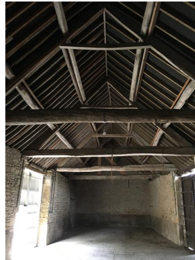
Plate 23: Main barn interior with tie beams and collars set beneath the upper tier of through purlins. All common rafters are replaced.
