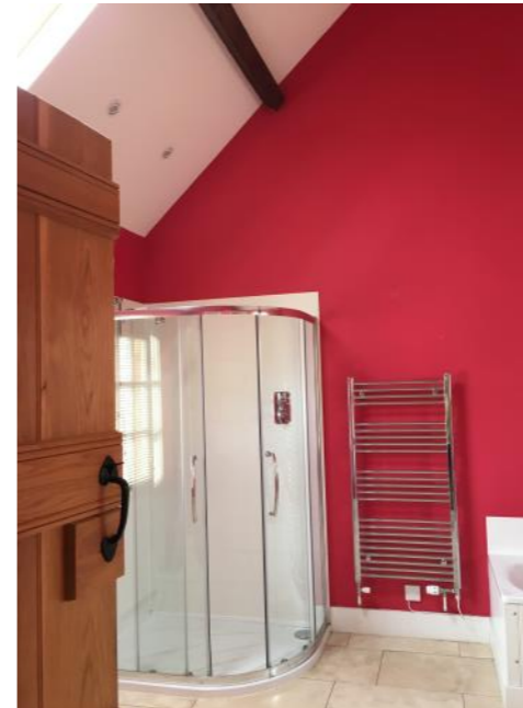
Plate 25: Modern bathroom inserted into eastern portion of the Victorian Extension and removing any heritage character or evidence of function.
