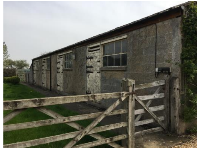
Plate 19: Building 17 concrete block structure to the east of the main yards. Doors and windows suggest possible stabling.
