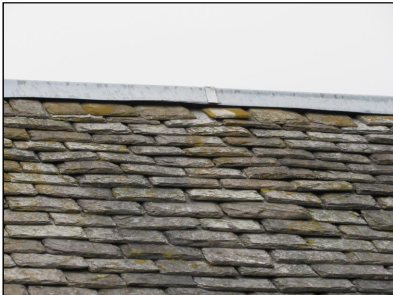
Figure 11. The void beneath ridge flashing is a common roost site for pipistrelle bats.
