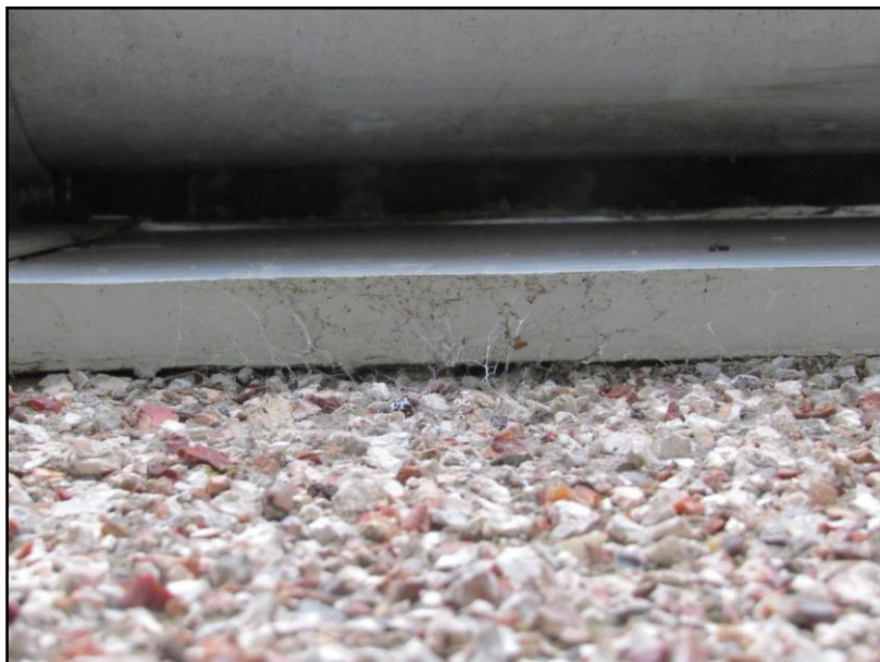
Figure 9. The fascia is tightly fitted to the render leaving no points of access for bat species around the eaves of the cottage.
