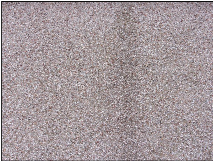
Figure 8. The external render is tightly sealed offering no points of access for bat species
