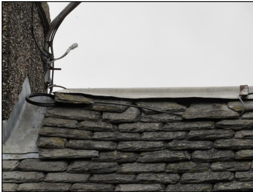
Figure 10. There are numerous gaps between and beneath the slates across the roofs of the cottage.
