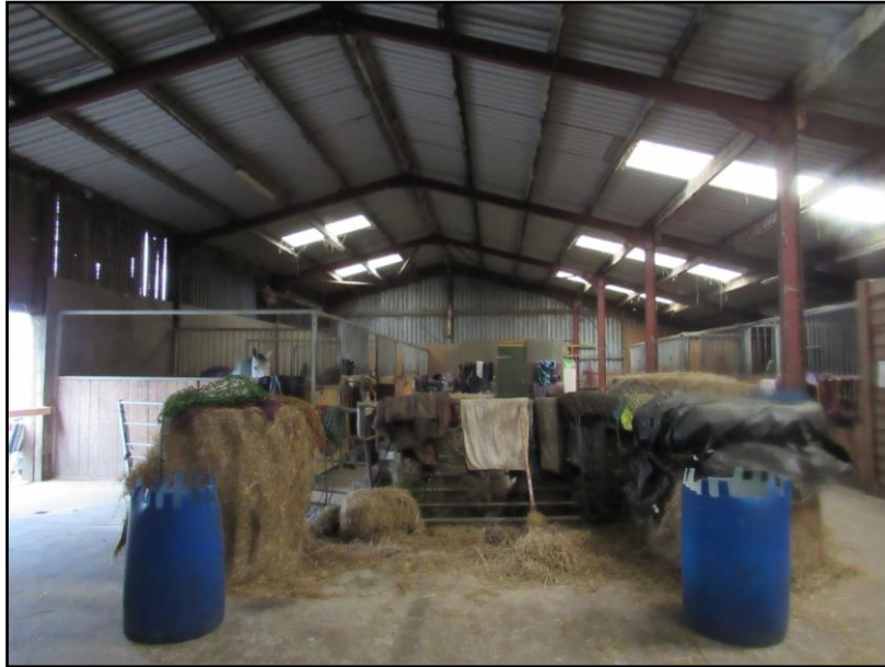
Figure 21. The interior of the shed is brightly lit and wholly unsuitable for roosting bats.
