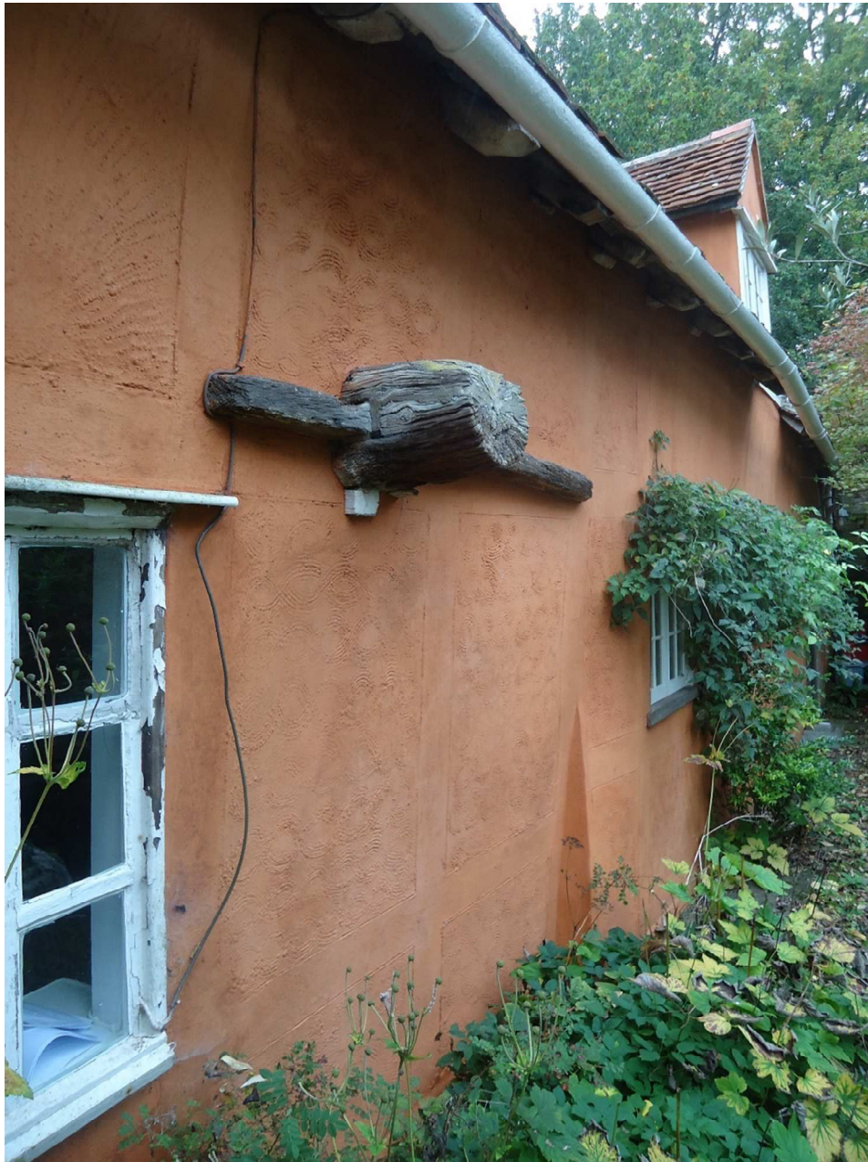
Figure 20: Needle beam protruding through the front wall of the hall.
