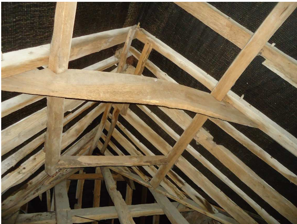
Figure 34: C17 clasped side purlin roof structure over the C16 and C17 sections of the house.
