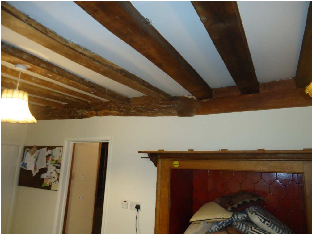
Figure 32: Part surviving bridging beam.
