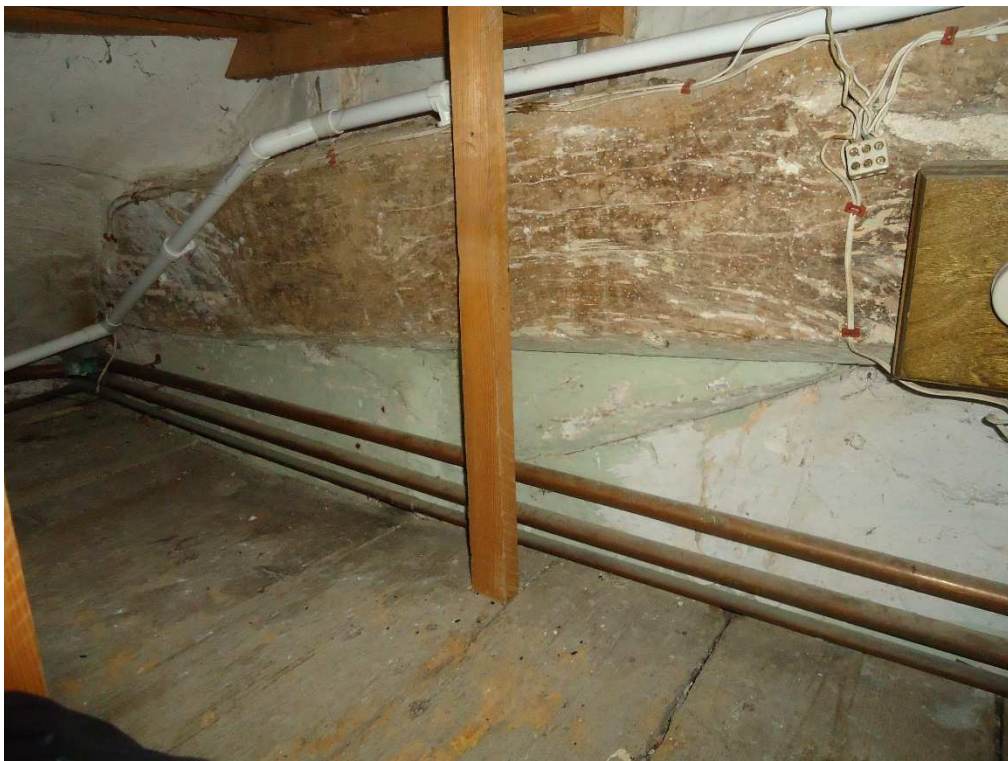
Figure 30: C16 brace in former open Truss 3.
