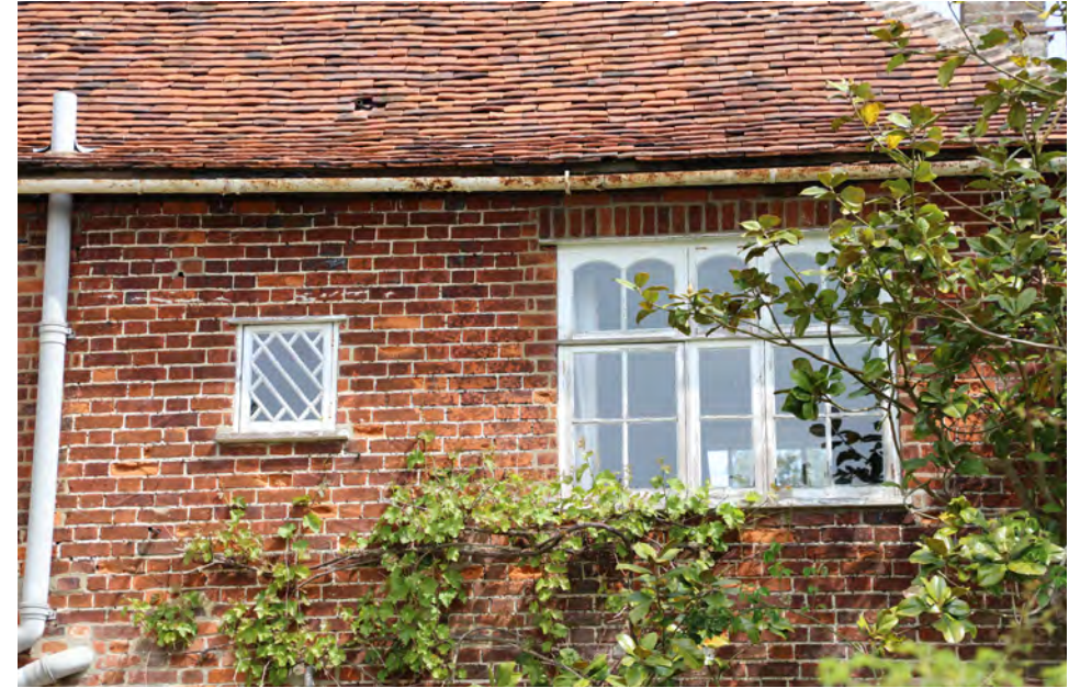
20th C inserted windows in south west brick elevation (RH window to be replaced)
