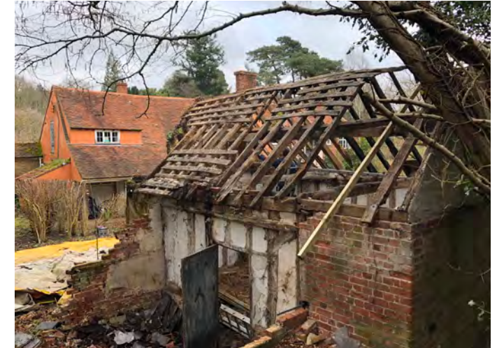
View of the existing Studio looking towards the north end of the house (which has been reinforced and protected with tarpaulin by the current owners)
