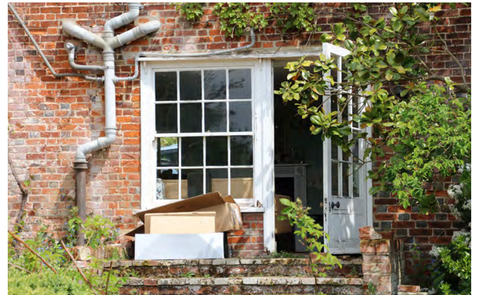
20th century window and door to be repaired. This area of altered brickwork to be covered by passage.
