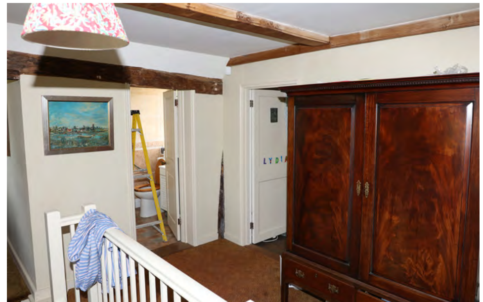
Chamber over Entrance Hall - modern stair, bedroom partitions and modern ceiling structure
