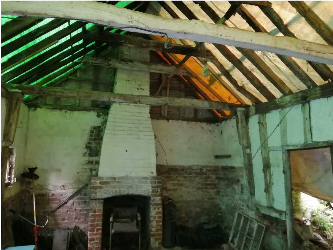
Photograph 9: Interior of the dilapidated outbuilding west of the house
