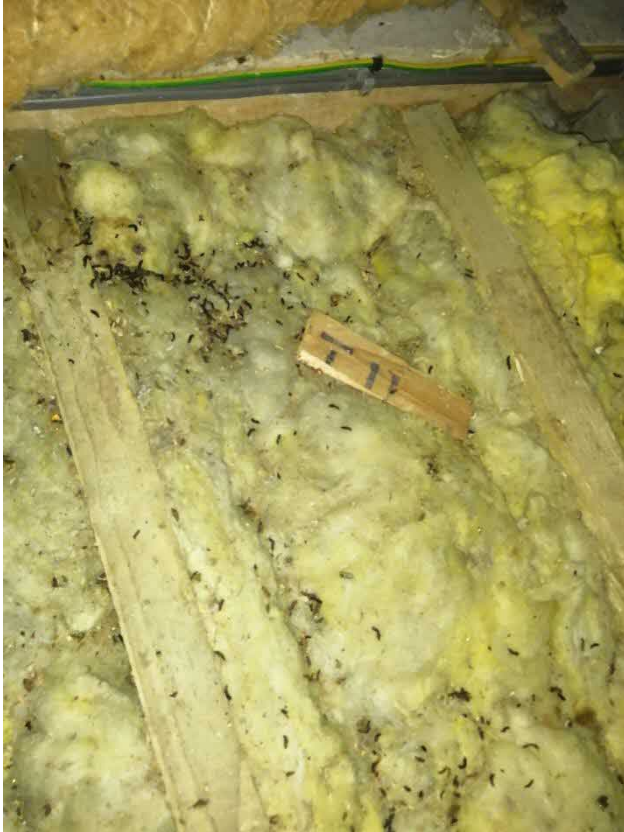
Photograph 5: Modest number of brown long-eared bat droppings in the east-central roof void
