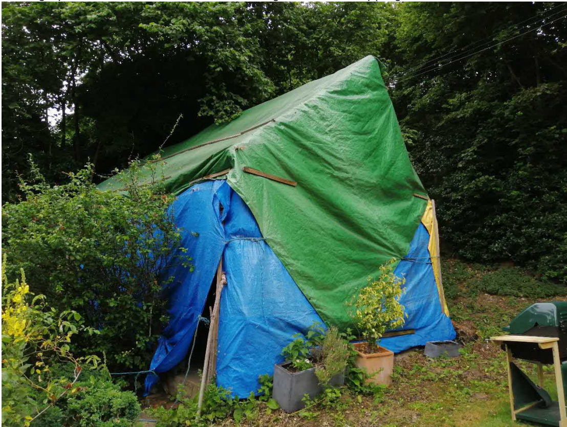
Photograph 8: Dilapidated outbuilding west of the house
