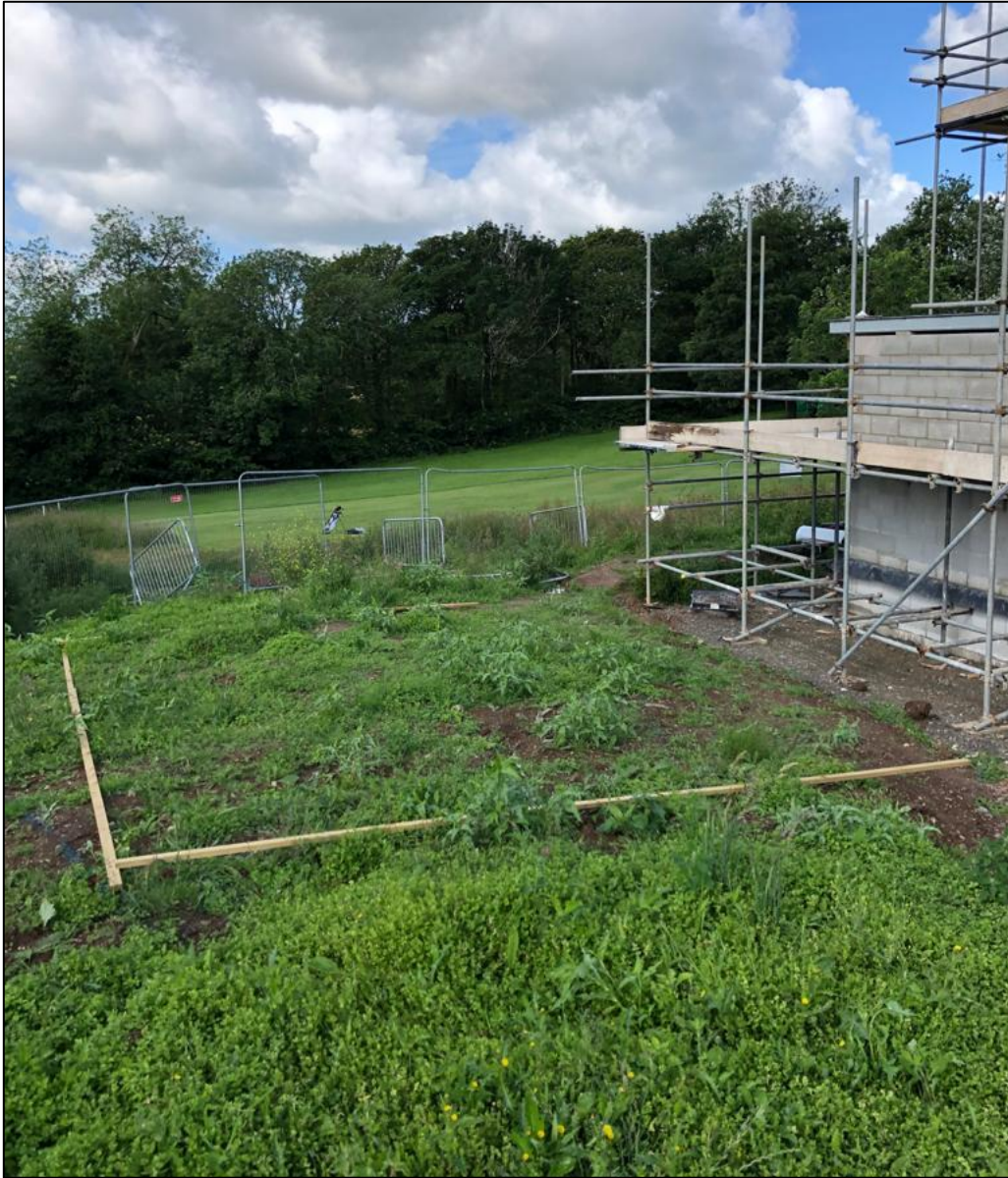
The view of the application site looking west towards the golf course with the land in question demarcated by the wooden planks
