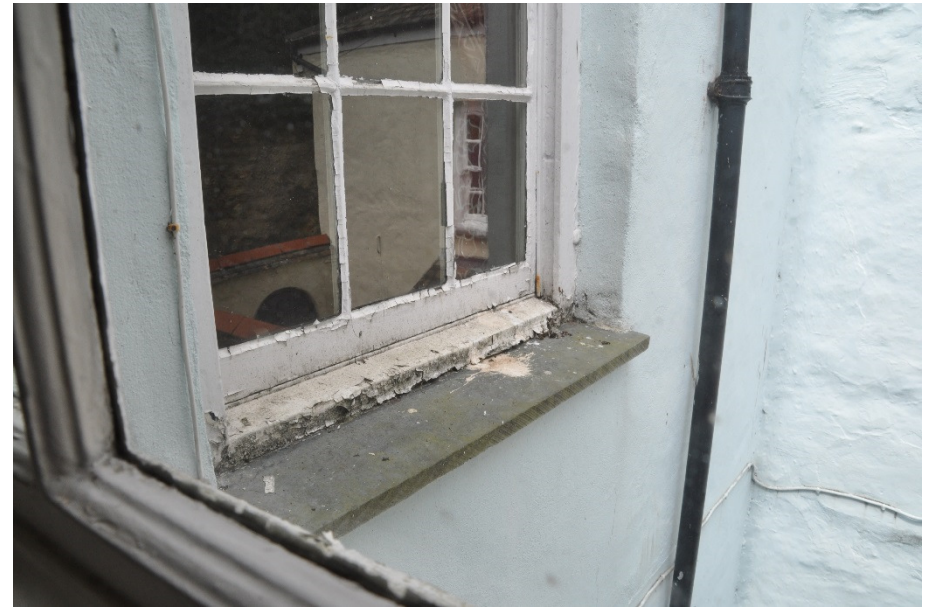
Fig 13: Significant deterioration to existing joinery noted.
