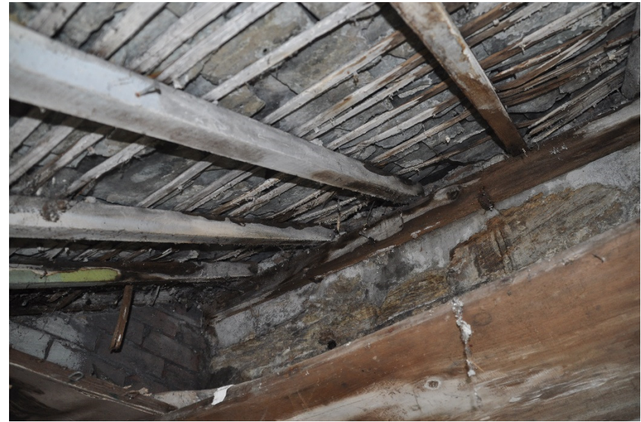
Fig 19: Significant moisture ingress to outbuilding and deteriorated roof.
