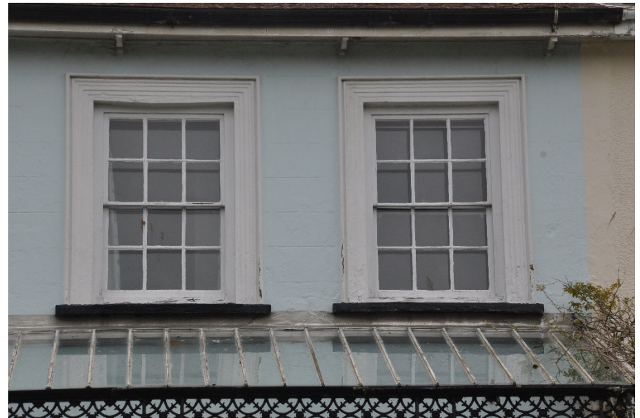
Fig 15: Modern veranda glazing bars in poor condition. Render mouldings around windows cracked and windows in poor condition.
