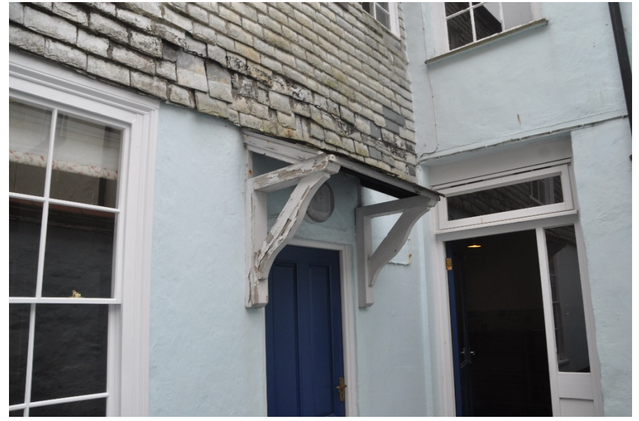
Fig 17: Defective slate cladding & defective modern porch canopy fitted with cement fibre roof slates.
