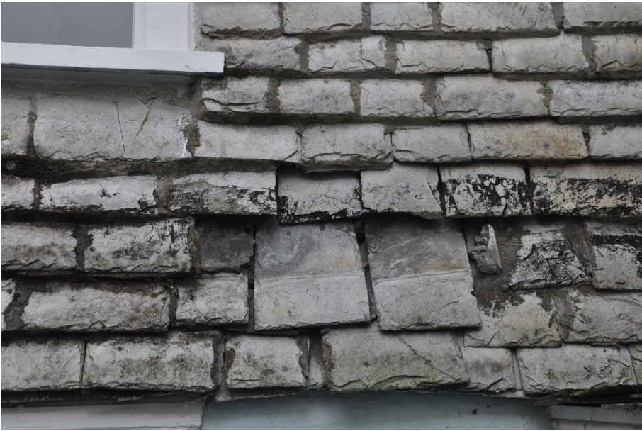
Fig 16: Significant defects and missing slates to rear range wall cladding.
