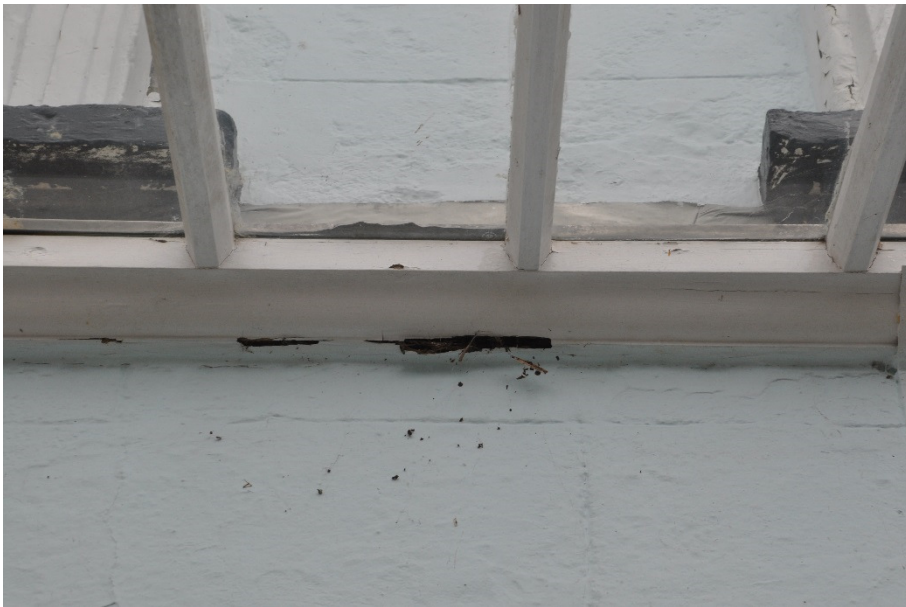
Fig 14: Modern veranda support timbers against existing wall significantly rotten. Abutment to wall covered by ad-hoc flashband repair.
