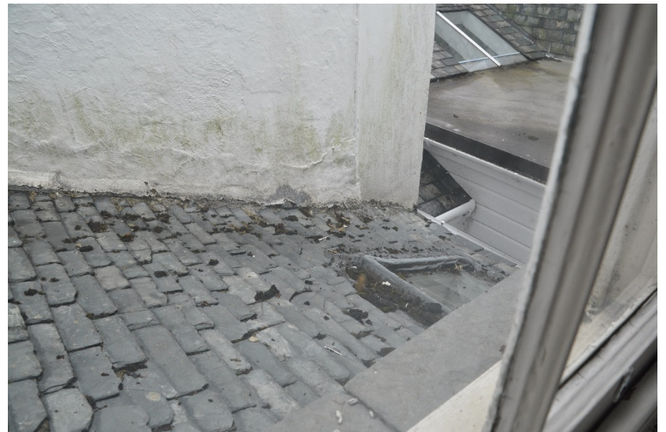
Fig 11: Existing roof over stair and roof window in rear range. Issues to flashings around window noted.
