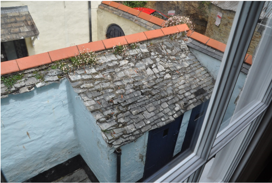
Fig 18: Significant defects to existing outbuildings.
