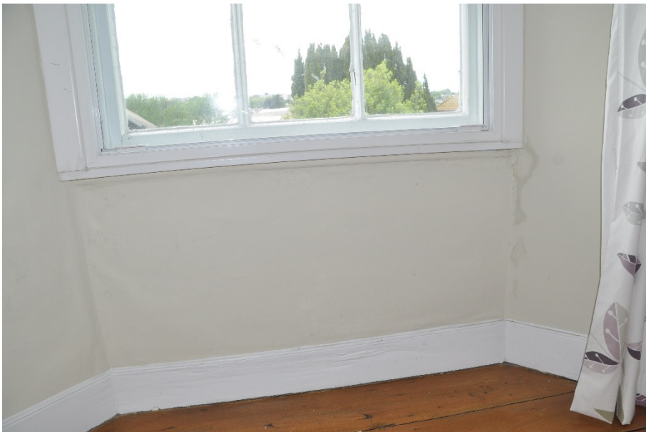
Fig 10: Existing main bedroom window. Window propped, secondary glazing installed and moisture ingress noted. Timber decay evident in skirting.
