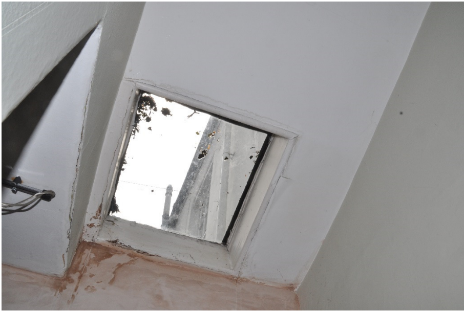
Fig 12: Existing roof window over stair- water ingress noted.
