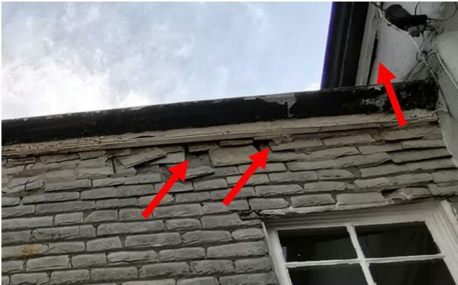
Photo 7. Showing the potential access points and roosting sites on the eastern side of the building
