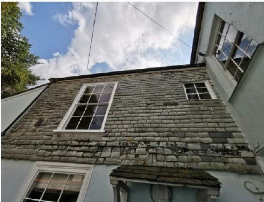
Photo 3. Showing the wall having slates on the rear extension
