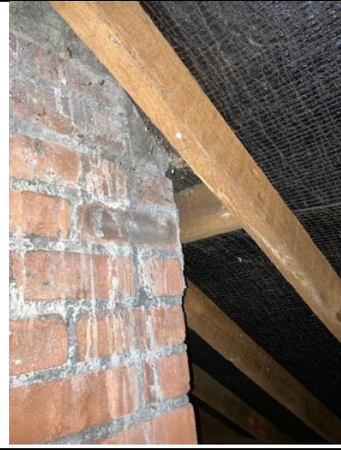
A.8 Small tear beside chimney
