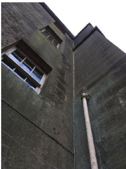
Existing Lightning Protection Down Conductor
