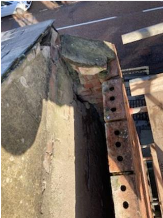
Photograph of unsafe brick skin at eaves interface
