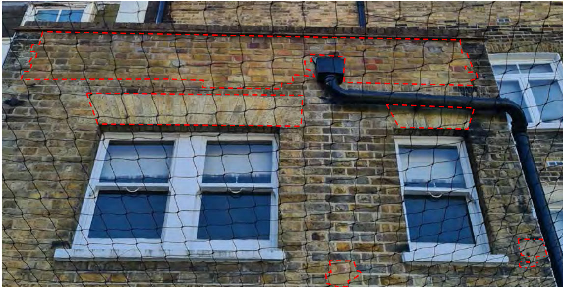
Figure 21: Detail: Patchy brickwork indicating history of alteration with poorly matched-in bricks
