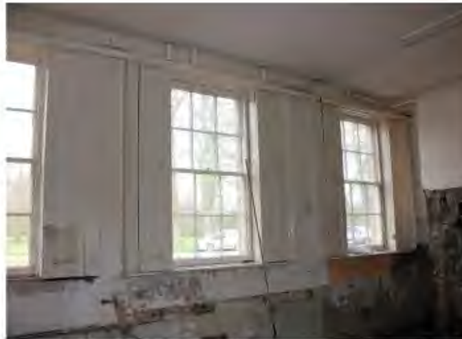
Shutter in former kitchen
