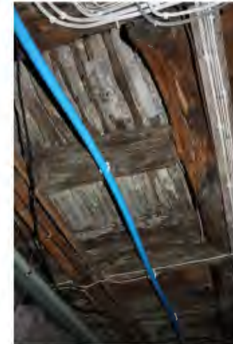
The underside of laths in the cellar plastered from above, providing evidence of a possible limecrete floor on the ground floor former service corridor in phase one
