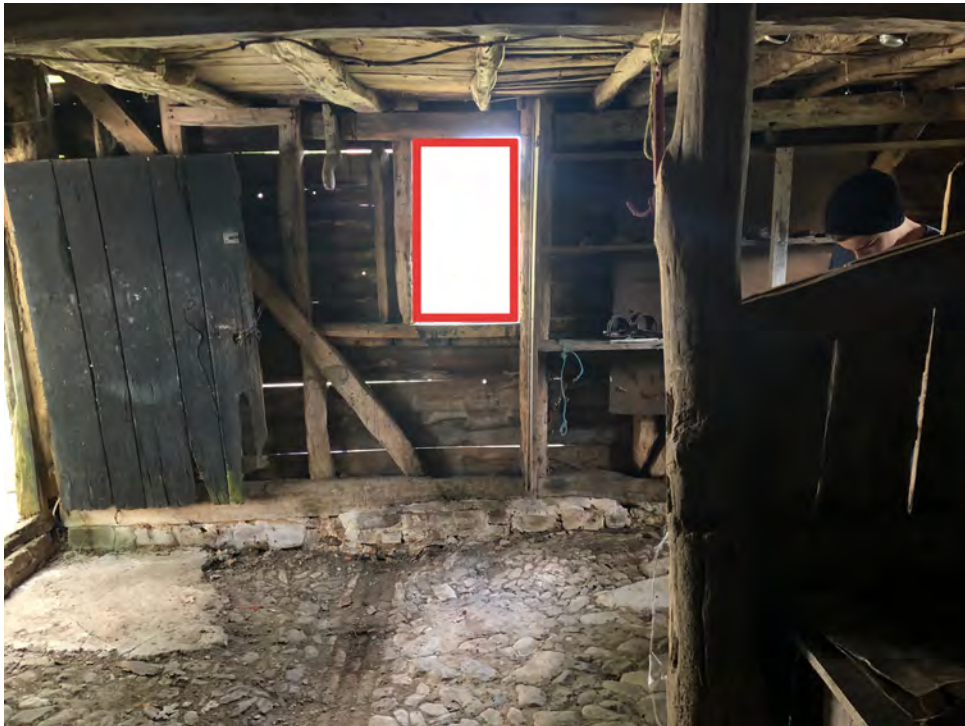
Barn interior – existing window opening to east elevation red box indicates area of new window in existing opening
