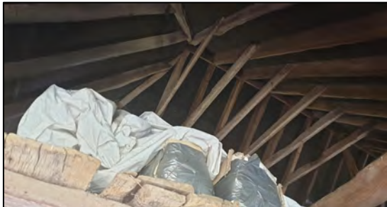
Photograph 3: The internals of building B3. Photograph taken by Tara Hall on 25 th March 2020.
