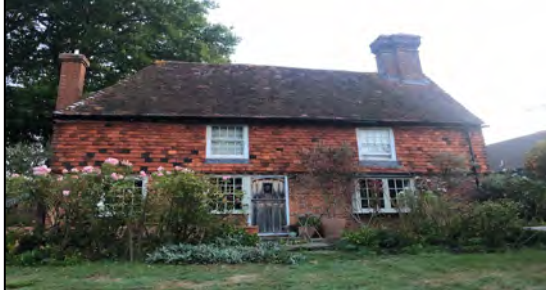
Photograph 1: The southern aspect of building B1. Photograph taken by Nicolle Stevens on 15th September 2020.
