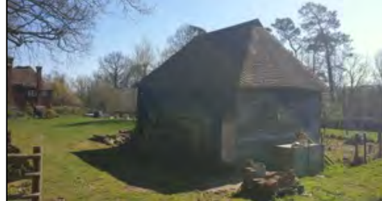
Photograph 2: The northern and western aspect of building B3 with western aspect of building B1 in the background. Photograph taken by Tara Hall on 25 th March 2020.
