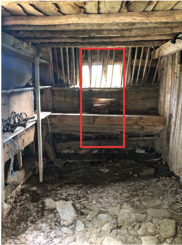
Barn interior – existing window opening to south elevation red box indicates area of new opening to the proposed glazed link
