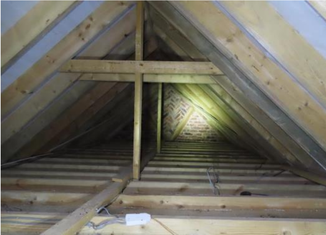
Photograph 9. Buildings at Church House Farm. Interior. View of part of the Building 3 roof-space. Looking south from north.
