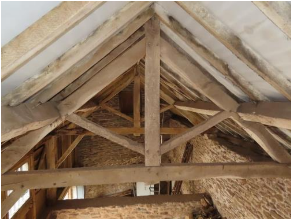
Photograph 8. Buildings at Church House Farm. Interior. View within the west part of Building 2. Looking west from east.
