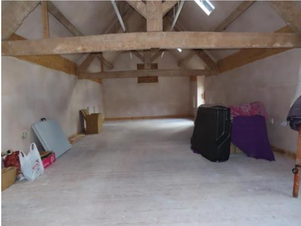
Photograph 7. Buildings at Church House Farm. Interior. View of the main (central and east-end) first-floor room of Building 1. Looking east from west.
