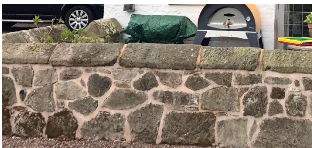
Figure 8.0 – Existing stone wall to be dismantled. The existing Sandstone is to be re-used in the new stone plinth.
