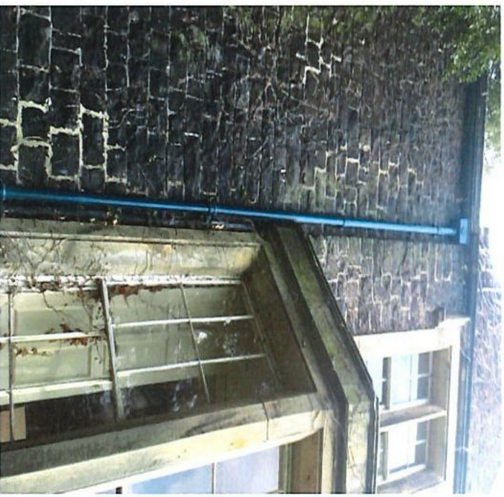
Vegetation growing through sashes and renewed rainwater pipe
