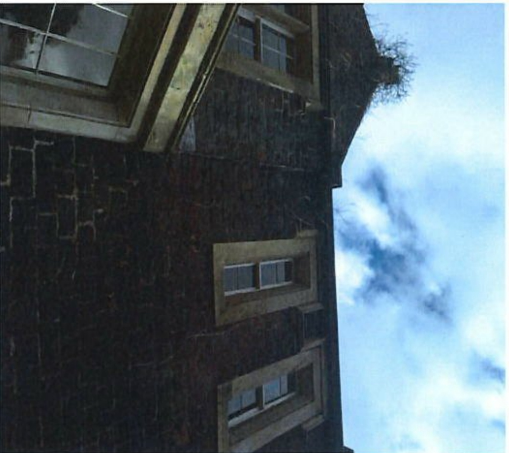
Vegetation to chimney Stack
