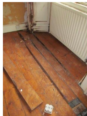
Damage to floorboards and panelling in North West bedroom
