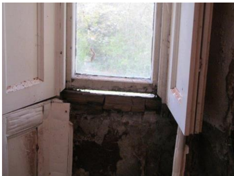
Damage to cill of main bathroom window
