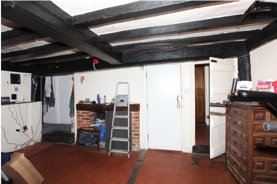
Illus. 9. The 20 th century fireplace in the living room with the massive binding joist of the 16 th century ceiling above. This joist spanned the approximate centre of the Tudor hall and is chamfered on both sides. Mortices are visible for large, flat-sectioned common joists at right-angles to the present joists. The storey post to the left preserves the outline of what may be a carved capital and attached shaft (illus. 11)
