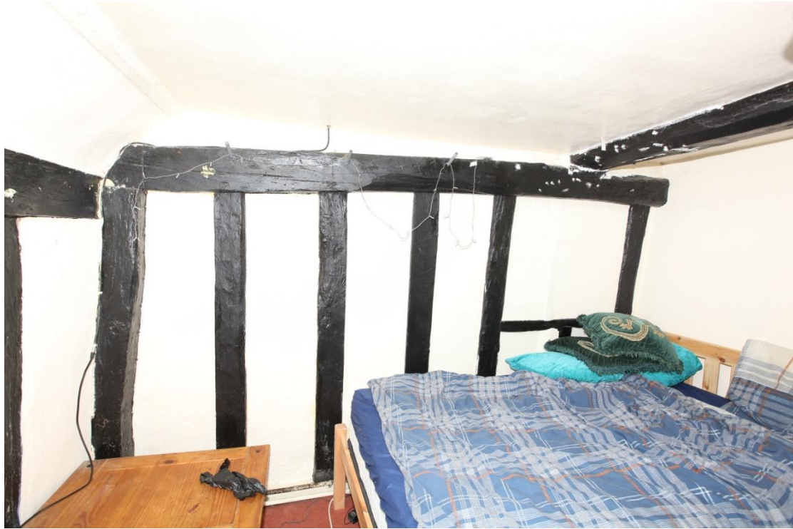
Illus. 15. The eastern gable of the hall chamber (i.e. the bedroom above the present living room). The wall studs are fully tenoned and pegged but the sill of the blocked central window is a nailed insertion and there are no mullion mortices in the fully exposed tie-beam above – because it occupies the position of an original door that opened into the missing service chamber.
