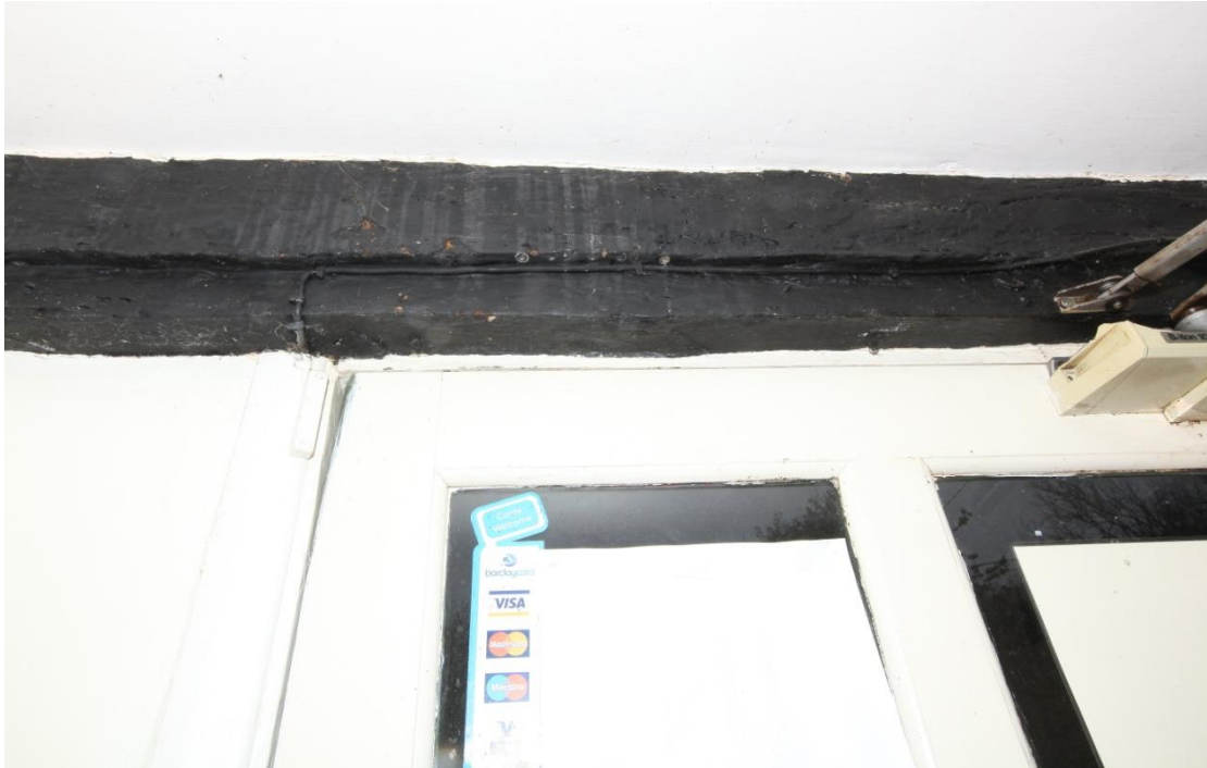
Illus. 6. The mid-rail of the 16 th century structure over the present northern entrance door showing the distinctive diamond-shaped mortices of the original window mullions in its underside with a rebate for a sliding shutter above. Only the triangular inner halves of these mortices are exposed, and a fillet of timber would have been nailed over the rebate to form a groove.
