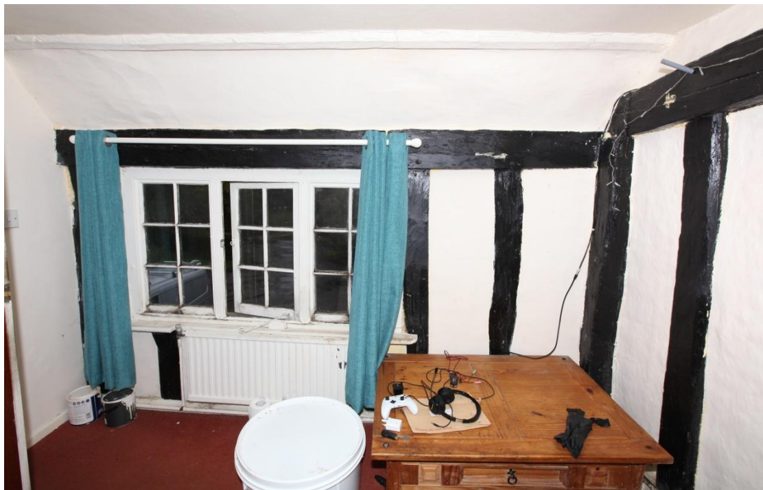
Illus. 16. The front wall of the bedroom over the living room showing a typical late-19 th century casement window with mortices for the diamond mullions of a 16 th century predecessor in the roof-plate above.
