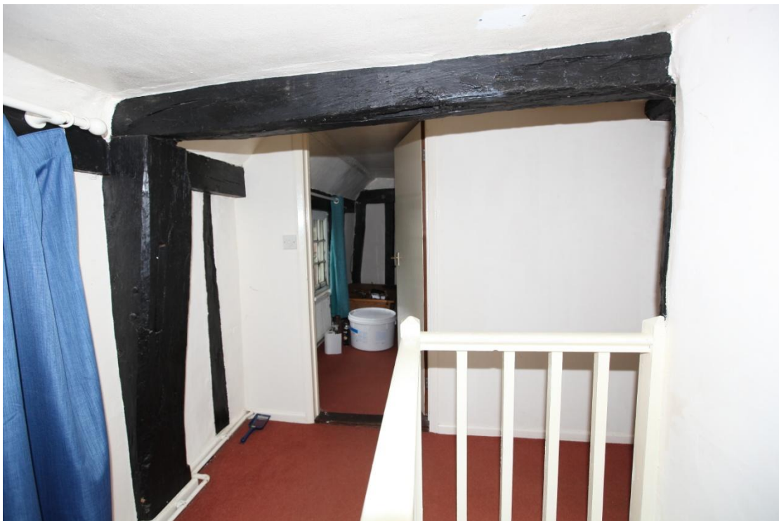
Illus. 12. The original tie-beam and heavy, jowled storey post of the hall chamber's open truss seen from the 20 th century stair landing in front of the rendered chimney to the right. Both the post and tie contain pegged mortices for a missing arch-brace matching the surviving brace to the rear (illus. 13).
