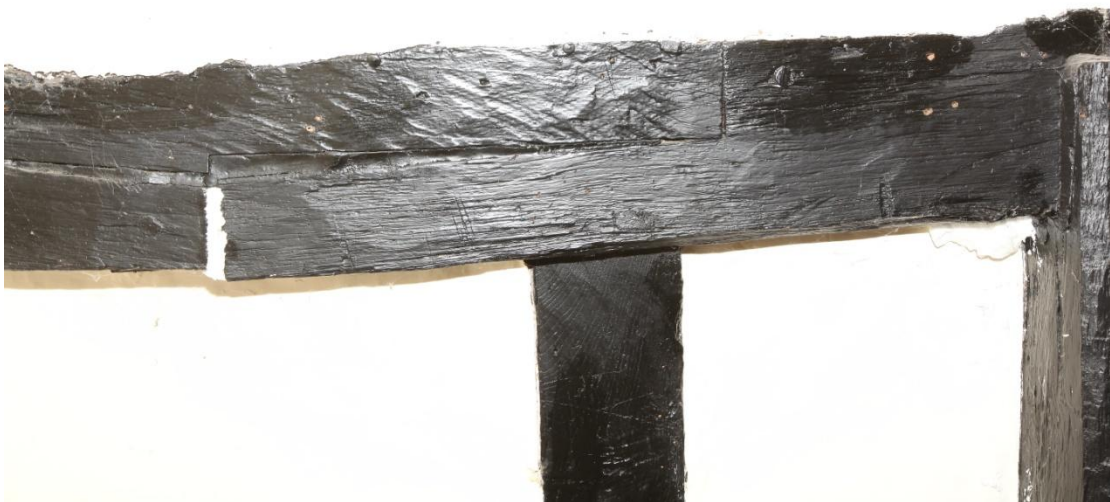
Illus. 18. A detail of the 16 th century edge-halved and bridled scarf joint in the rear roof-plate (as shown in illustration 16). Joints of this kind were superseded by face-halvings around the turn of the 17 th century.
