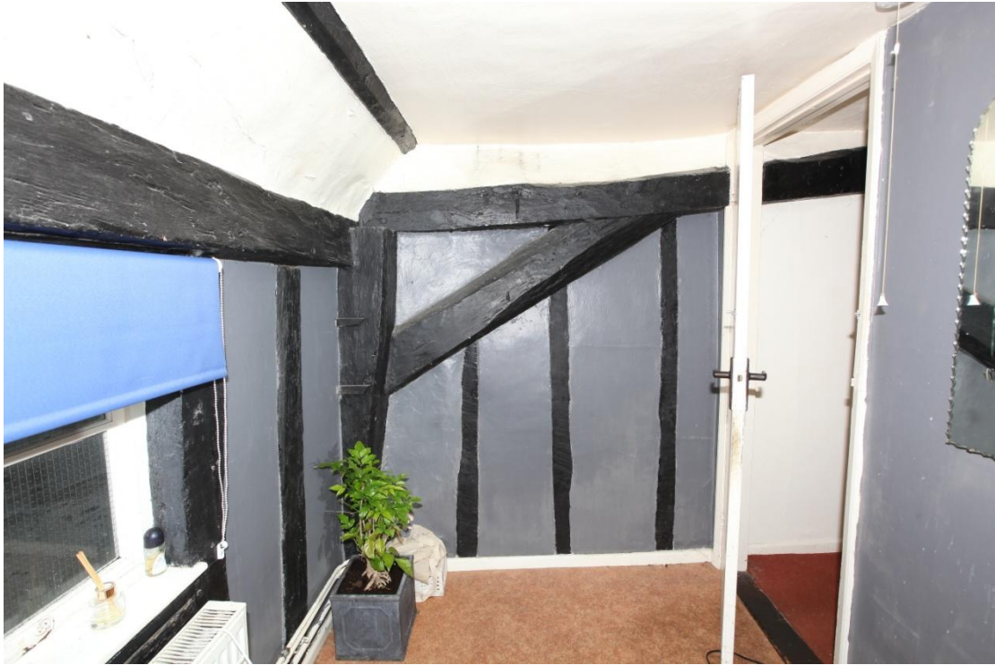
Illus. 13. The intact 16 th century arch-brace to the rear of the original hall chamber's open truss, seen from the east. The narrow studs are likely to have been inserted along with the chimney in the 17 th century. Mortices for diamond mullions are visible in the roof-plate above the present window to the left (illus. 13).
