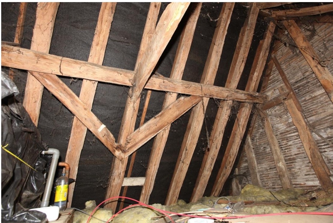
Illus. 20. The western end of the roof structure, with the gable to the right. This clasped-purlin structure could survive from the original 16 th century house but its nailed wind-braces suggest it was rebuilt as part of the 17 th century remodelling. Identical nailed braces survive in the front wall immediately opposite.
